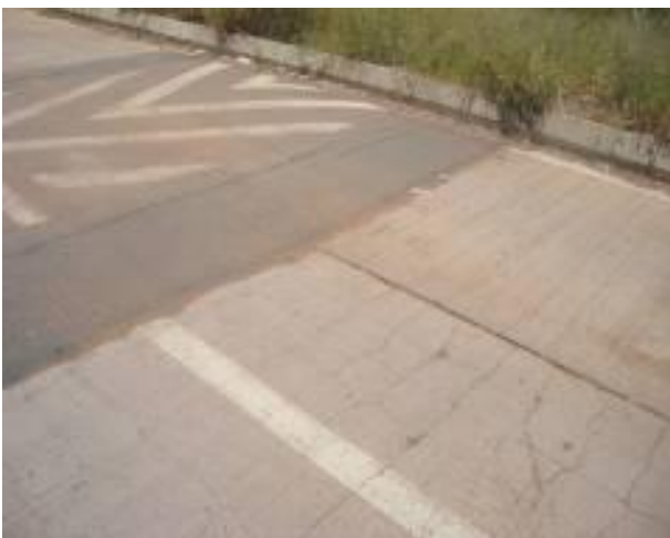
Photo 3 - Block cracks on CSIR test at Mamelodi
