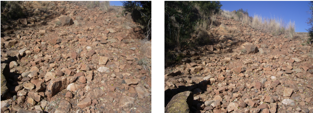
Picture 4: loose stones that needs to be stabilized. Source: M.Molibeli ,June 2007
