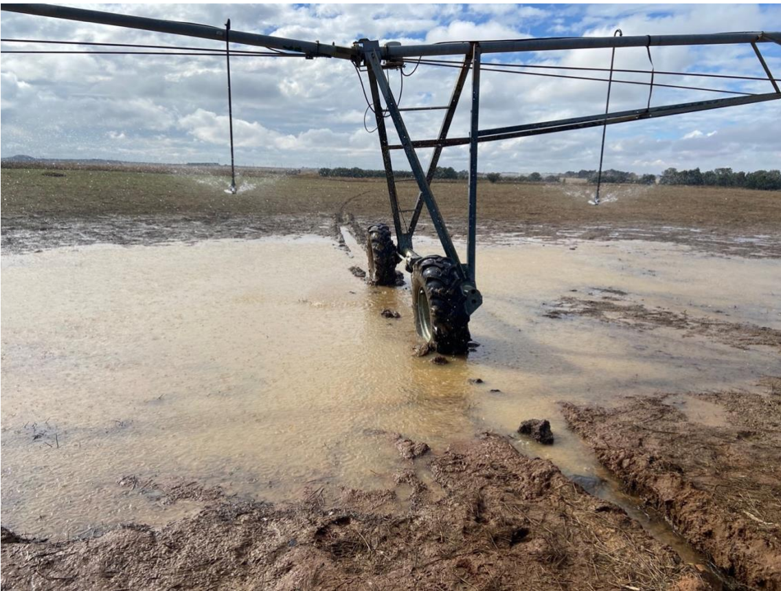
Figure 7.4: Water ponding due to surface subsidence and insufficient filling
