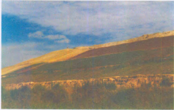
FIG. E.7 - Study site I. Rehabilitation of the slope wall to prevent wind erosion and dust generation.
