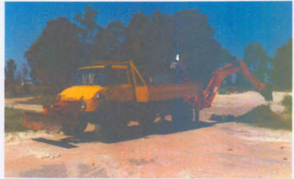
FIG. E.8 - Track-mounted backactor on a Mercedes Unimog in action at one of the investigated sites.
