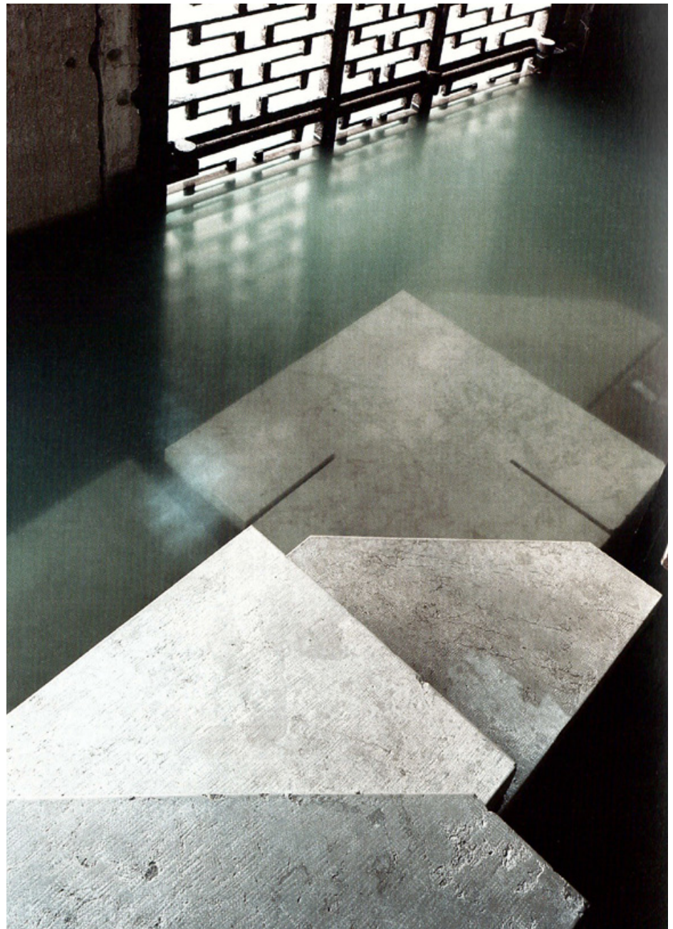
Fig. 5.20 Photograph showing the occurrence of flooding along the building edge. Photograph by Chemollo, A (2003).
