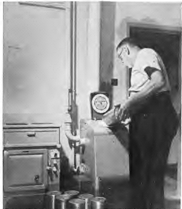
Stoking up a modern boiler with carefully measured and analysed quantity of fuel.
