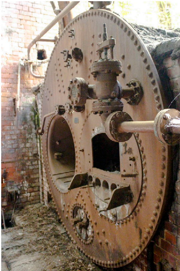
Fig 195 Boiler to be hung in central space
