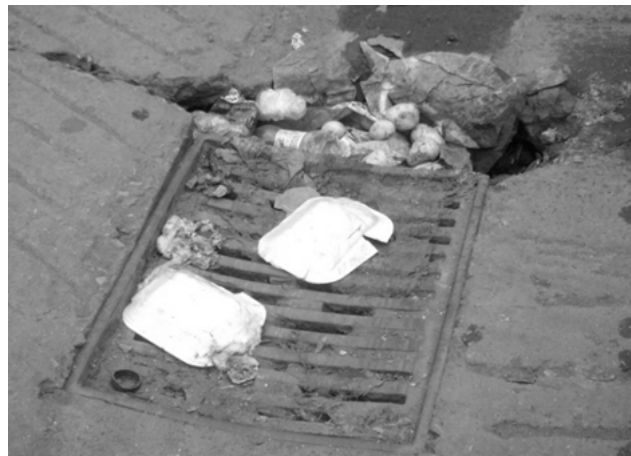
Fig 3.07 Block stormwater drains also affect the communities wellbeing and security.
