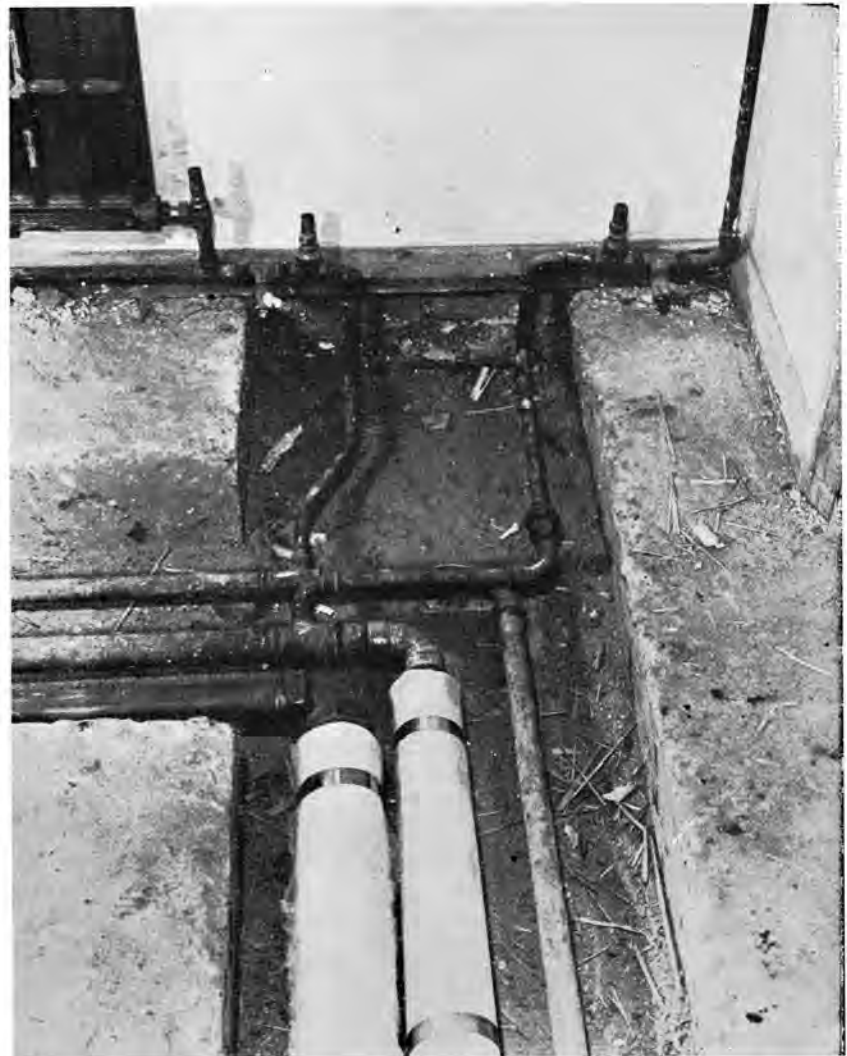
PIPE LINES FOR HOT WATER.
