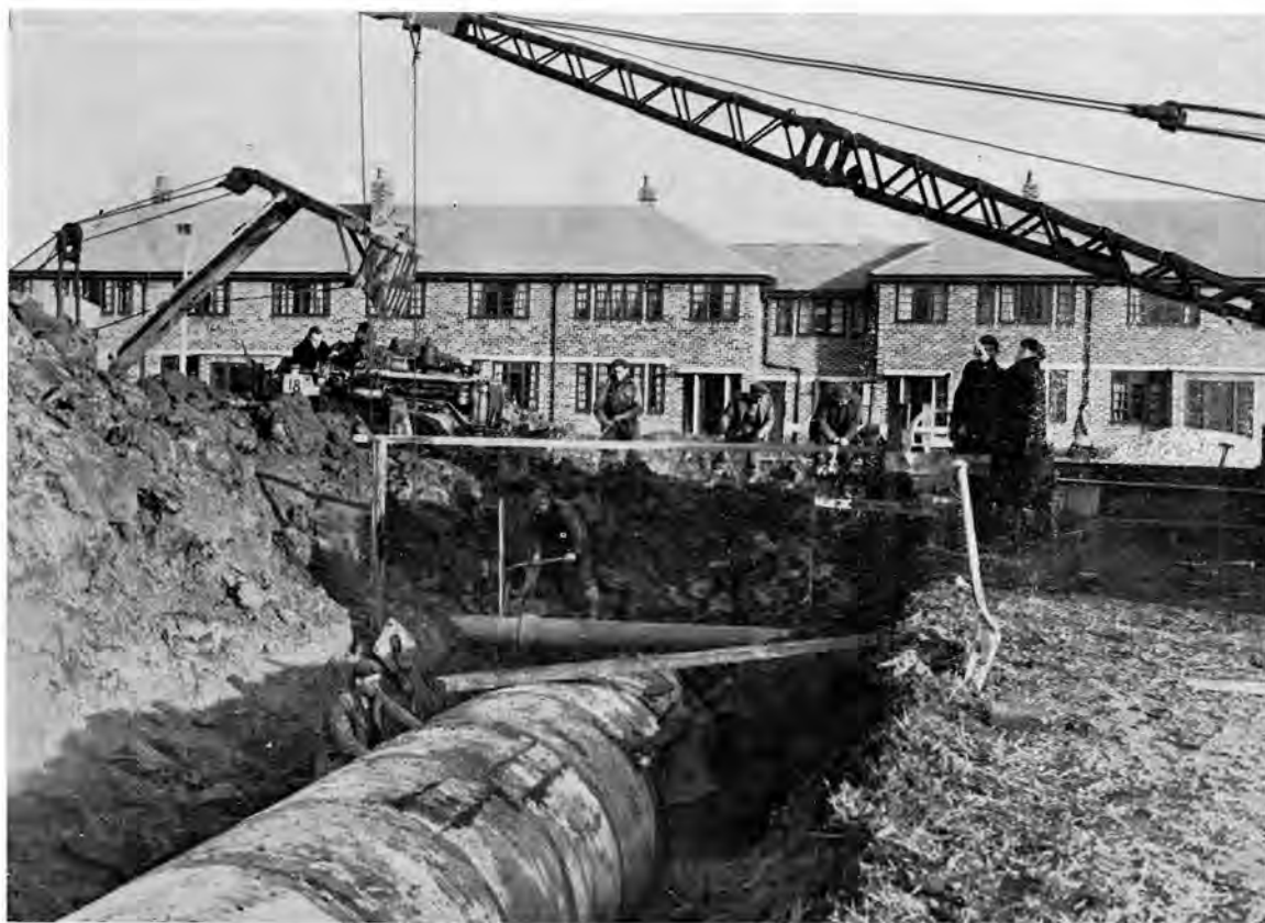
ILLUSTRATION SHOWS THE CULVERT BEING DUG. The concrete sections house the glass fibre lagged hot water pipes, and adequate room is provided for inspection purposes.
