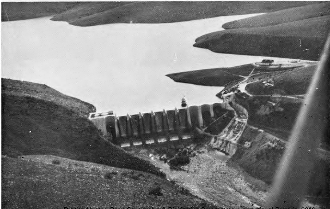
(Bottom) VIEW LOOKING UPSTREAM DURING A STAGE IN THE CONSTRUCTION OF THE DAM.
