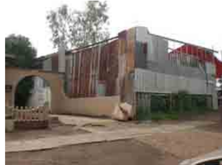
fig. 02_ Decaying urban environment, Buitenkant Street
