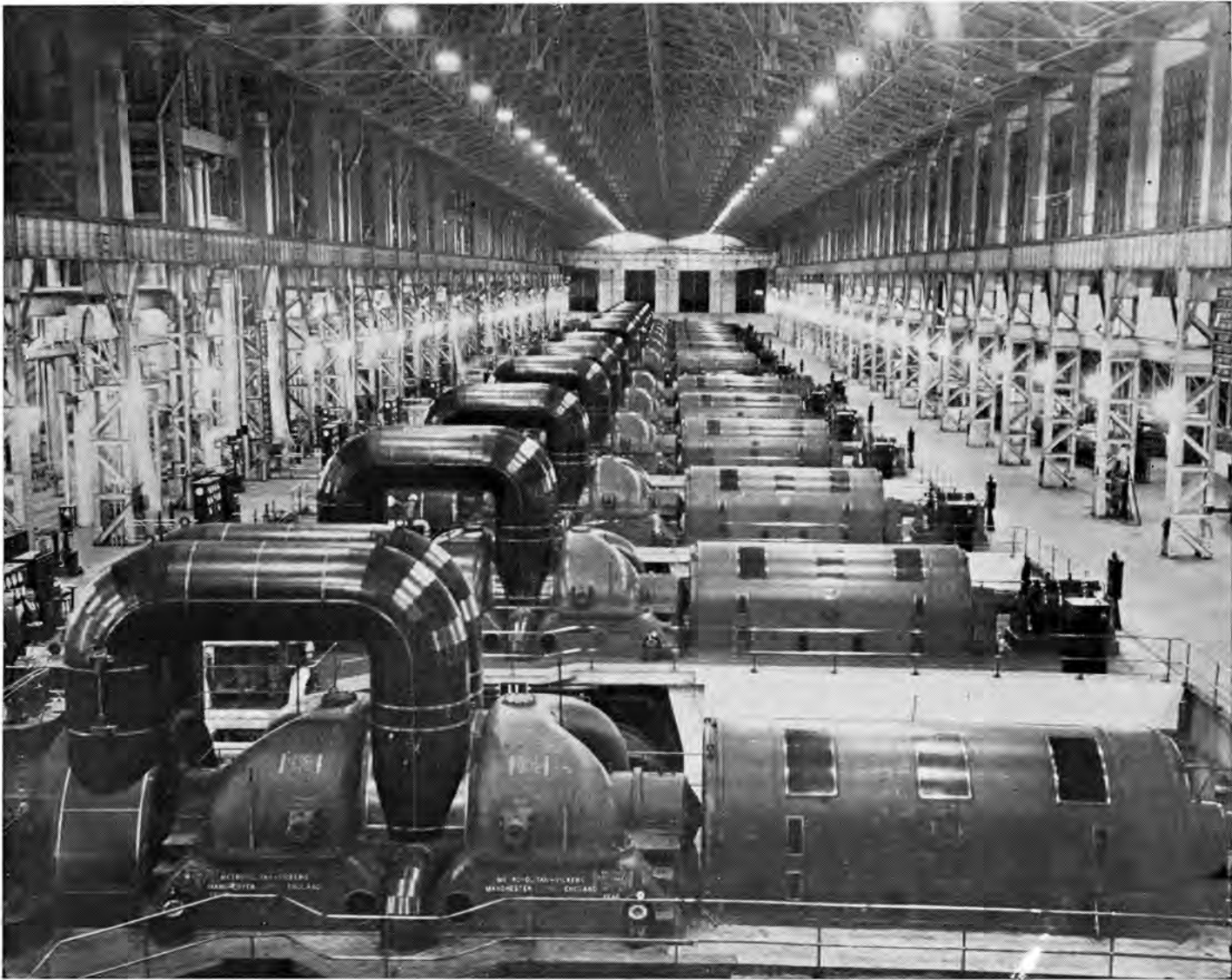
The Klip station interior, showing the twelve 33,000 kW turbo-alternators in operation.
