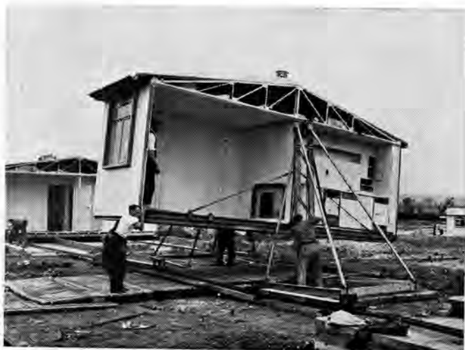
A house, pre-fabricated in Britain, about to be erected on a site.
