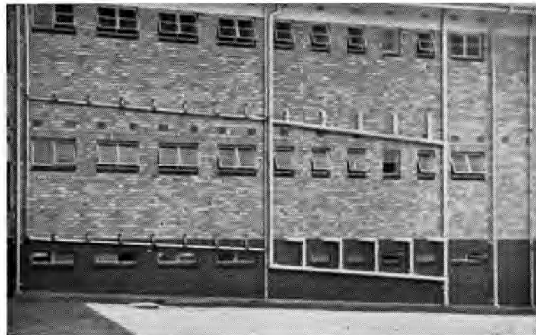
External details of the piping from the lavatories, baths and wash-basins in the girls' block, south wing.
