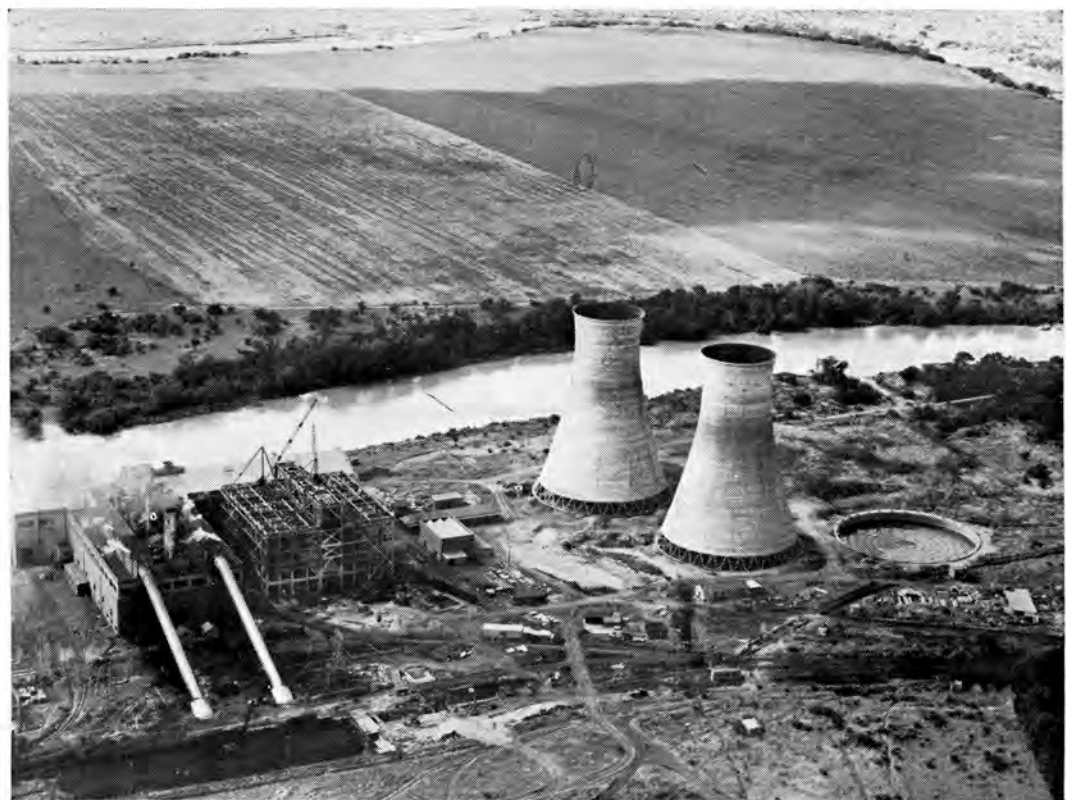
The Colenso power station, the main Natal installation, where a second station is now under construction.
