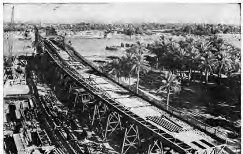
The first railway bridge, ever to span the River Tigris, now approaches completion.
