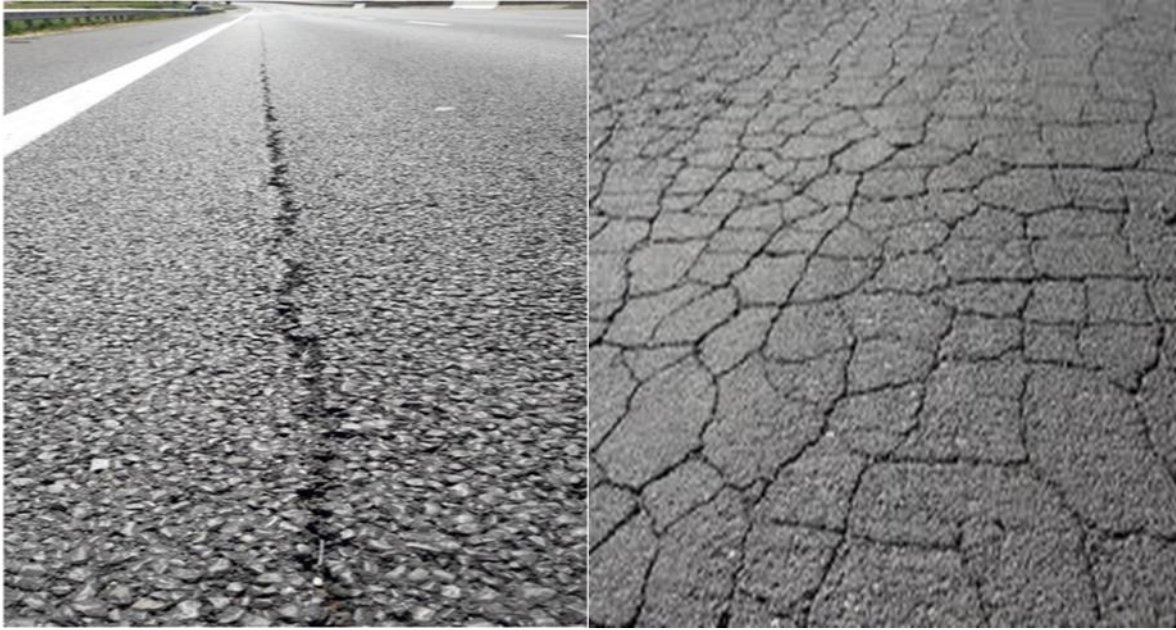
Figure 2-1: Examples of fatigue on asphalt pavement
