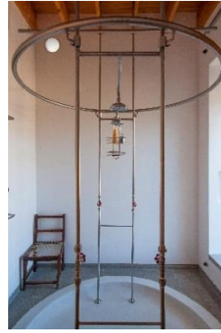
Figure 76: The exposed piping of the shower. (Wolff Architects, 2024:online)
