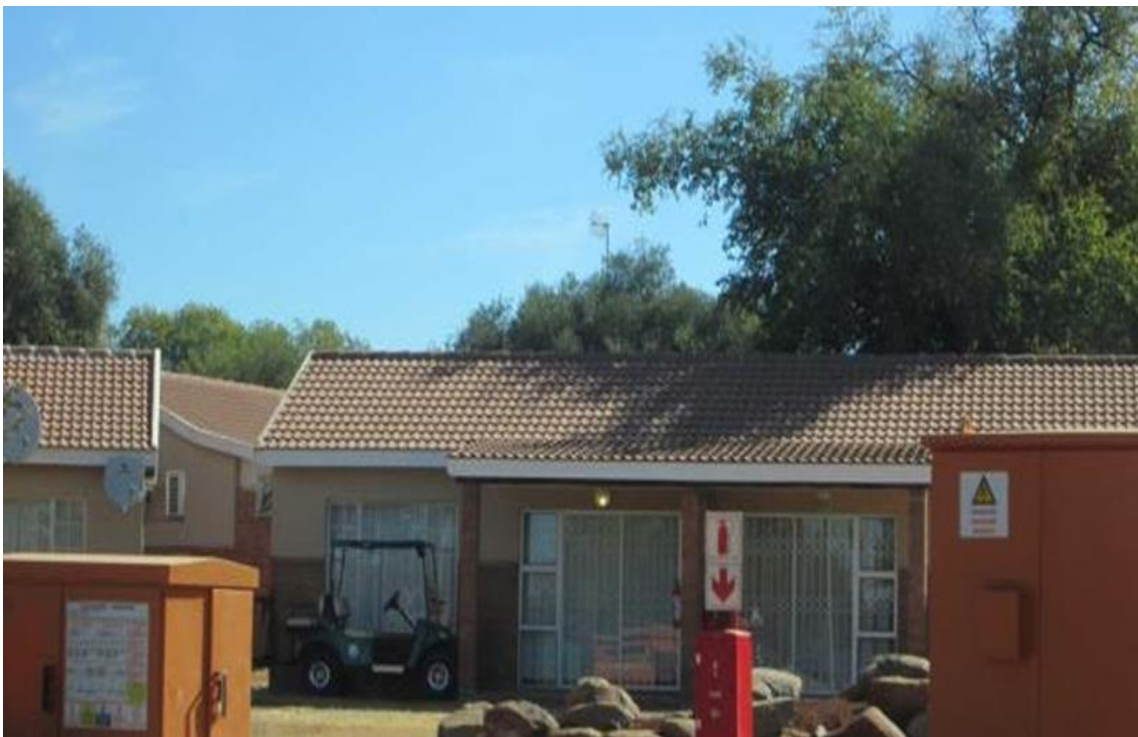
Figure 6.37 Single quarters with a private power substation independent from unreliable municipal power supply
