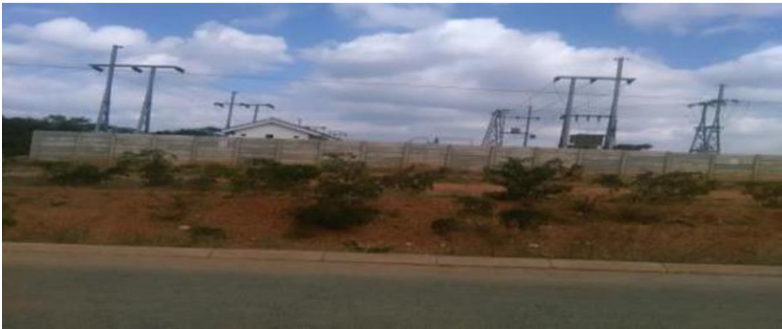
Figure 7.18 The 33 kV substation installed by Unki mine to supply power to their Impali houses
