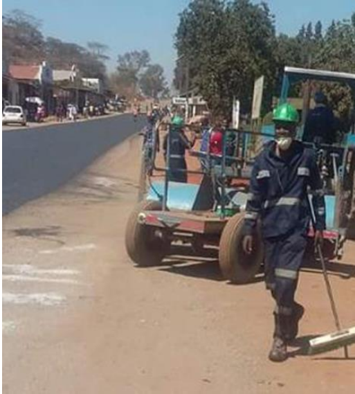
Figure 7.12 Main street in Shurugwi CBD. Shurugwi Town Council workers are resurfacing a section of the main street damaged by trucks and heavy machinery from the mine.
