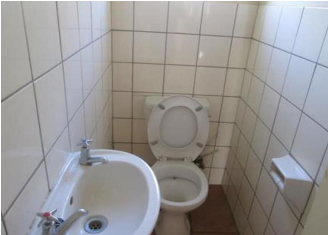
Figure 6.8 Mlanje SAV: Toilet and basin with hot- and cold-water taps
