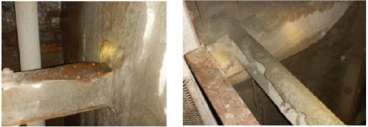
Figure 5.3: Bunton impact damage on buntons from falling objects
