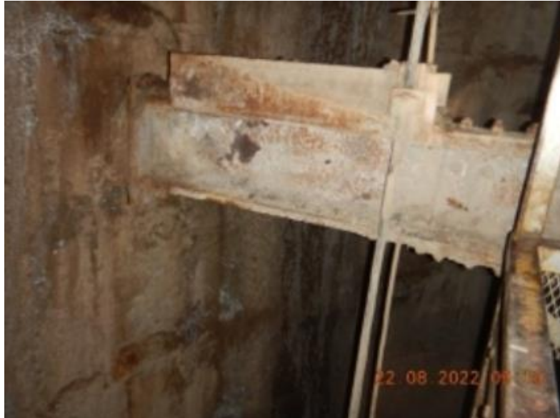
Figure 4.6: BUN-02 Set 5 recently corroded through
