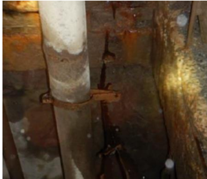
Figure 4.5: Pipe supports severely corroded
