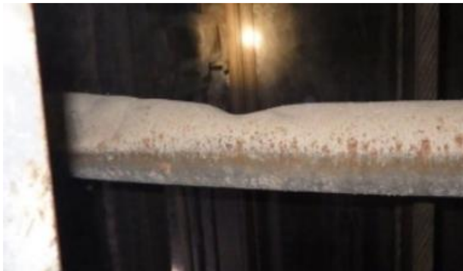
Figure 4.12: Impact damage example (Cat. 3)
