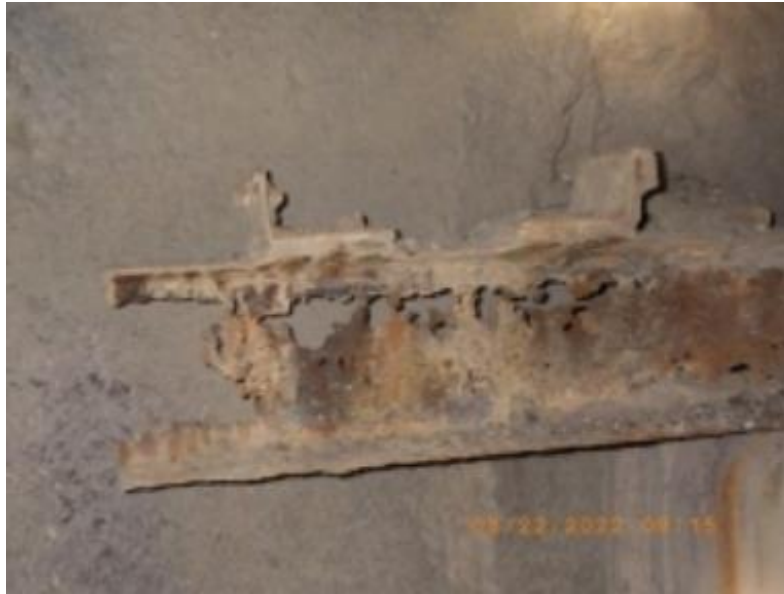
Figure 4.7: PST-04 set 33 severe corrosion
