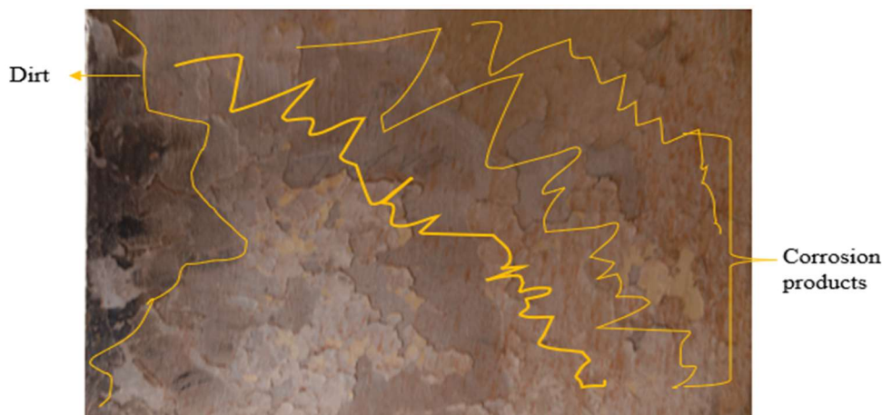
Figure 32: The amalgamated corrosion products on the North wall. Photograph by author.
