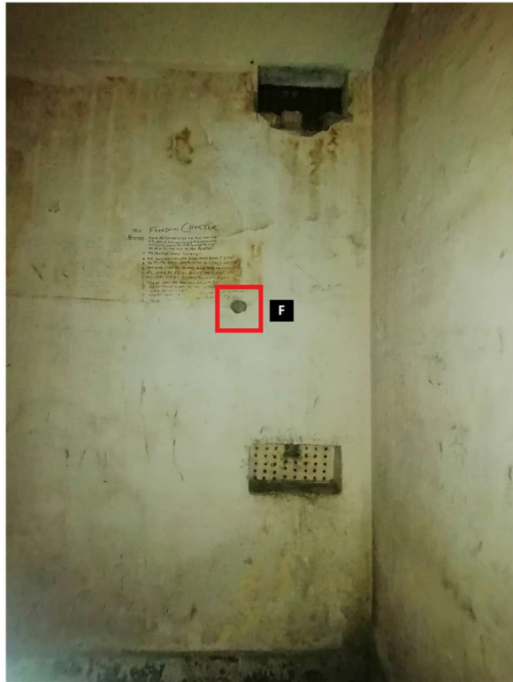
Figure 17: Area of Loss, lacuna 6. South wall. Photograph by author.
