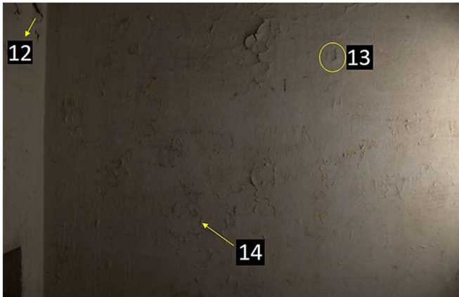
Figure 24: A cluster of deteriorations on the West wall. 2023. Photograph by the author.
