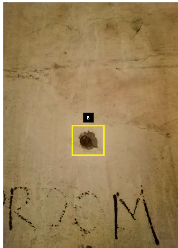
Figure 15: Area of loss, lacuna 4, South wall. Photograph by author.
