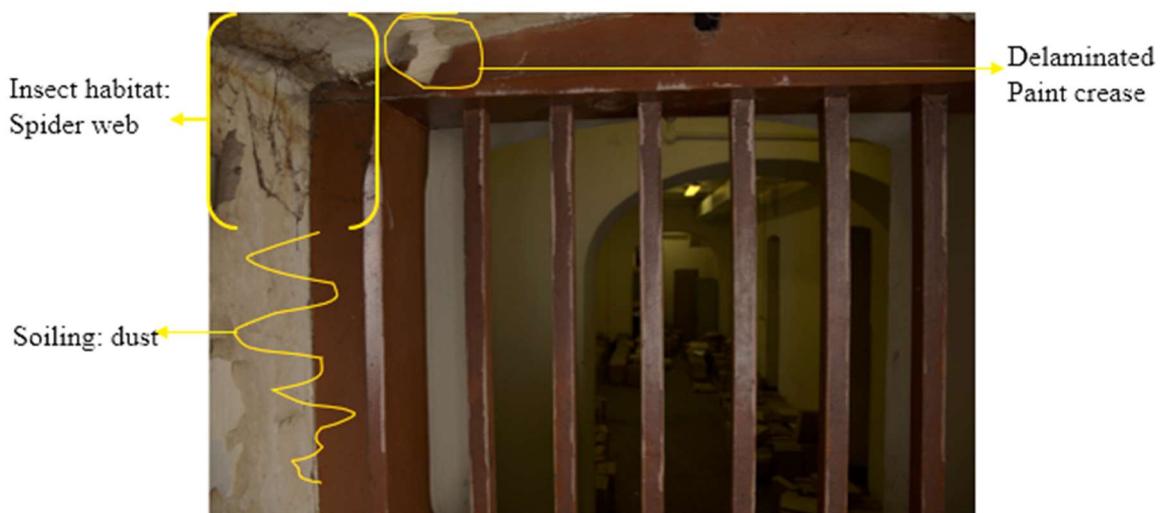
Figure 41: Biological deterioration on the North wall. Photograph by author.
