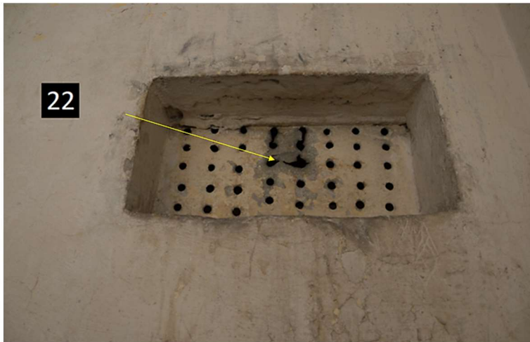
Figure 39: Deteriorations on the South wall ventilation panel. Photograph by author.
