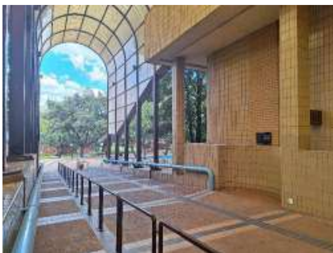
Figure 30: Extensively long entrance ramp of museum building, with no landings. The light blue hand rails are not grabbable and are covered in bird droppings, while the small, brown ones are an afterthought that limits use to a separate area.
