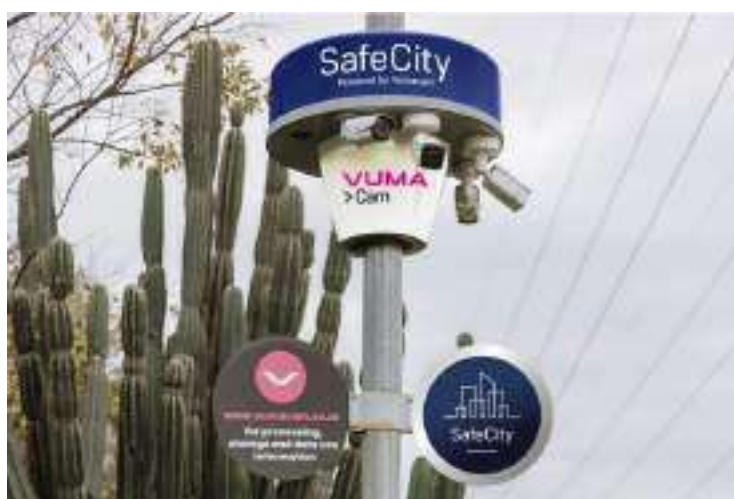
Figure 32: ‘SafeCity’ surveillance cameras installed across Tshwane (VumaCam 2023)
