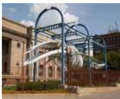
Figure 35: Arched frame installation at the Natural History Museum, Tshwane (SA History n.d.)
