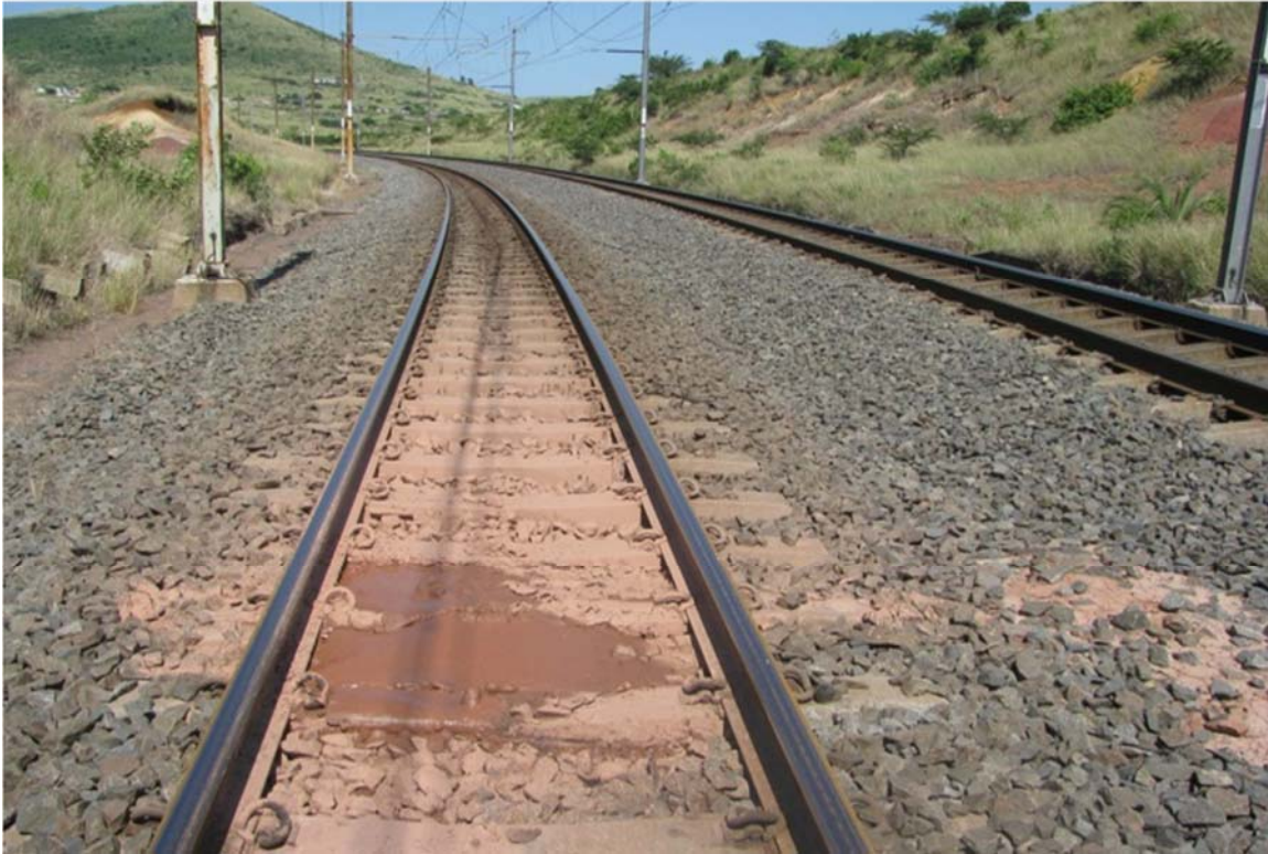
Figure 1-1: Railway track with poorly performing formation (Coal line, Empangeni)
