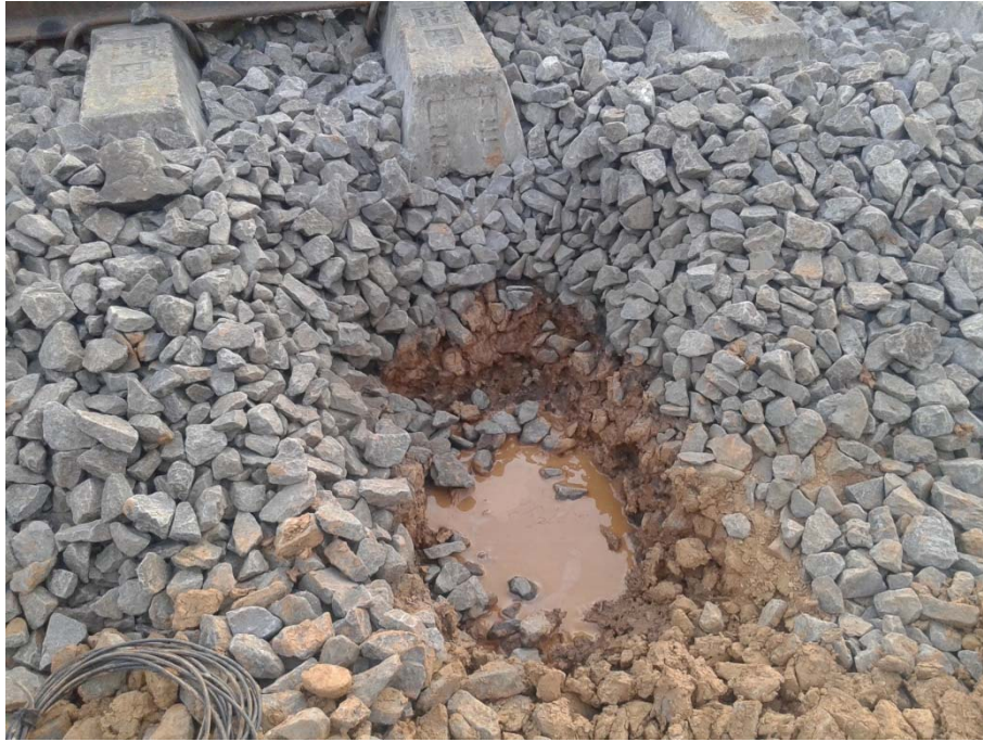
Figure 3-9: Increased moisture during the testing (Izolof - March 2015)
