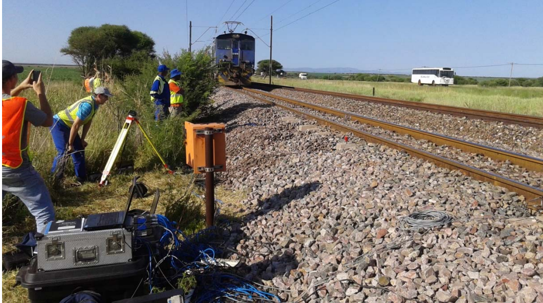
Figure 3-4: Overview of track at Amandelbult with instrumentation ready for data collection
