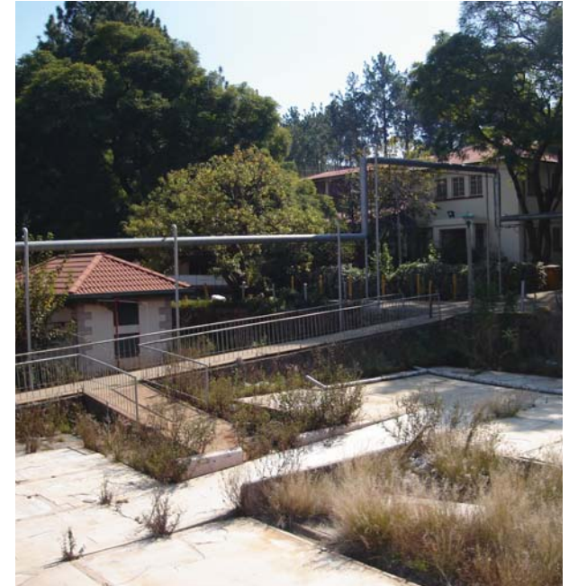
Fig. 3.21: Remains of demolished buildings (2008 and Author, 2008)
