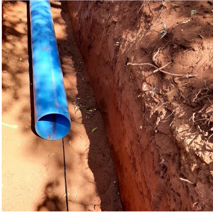
Figure 3.11. Photograph showing the position of the FO cable relative to the laid pipeline.
