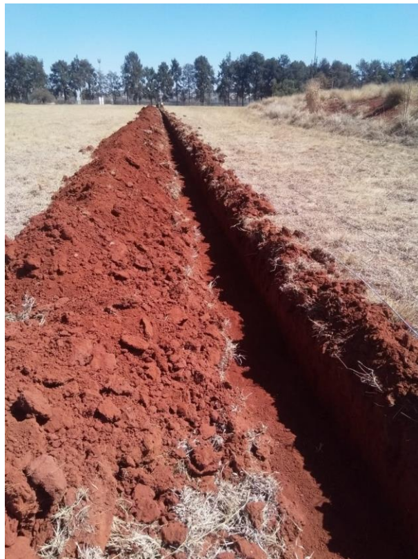
Figure 3.2. Standing point view of the trench prior to installation of the fibre optic cables.
