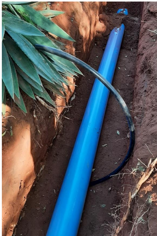
Figure 3.12. Photograph of one of the standpipes leading down to the level of the FO cable installed along the pipeline laid in Tom Jenkins Drive.
