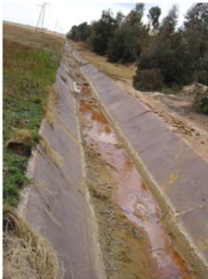
29 SOLUTION TRENCH CONVEYING CONTAMINATED WATER
