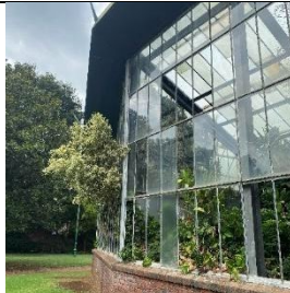
Figure 61: Plants growing through the broken greenhouse.
