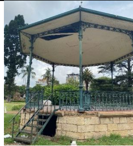
Figure 58: Current Victorian-style bandstand with broken roof and balustrade
