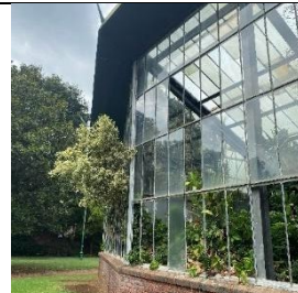
Figure 51: Plants growing through the broken greenhouse.
