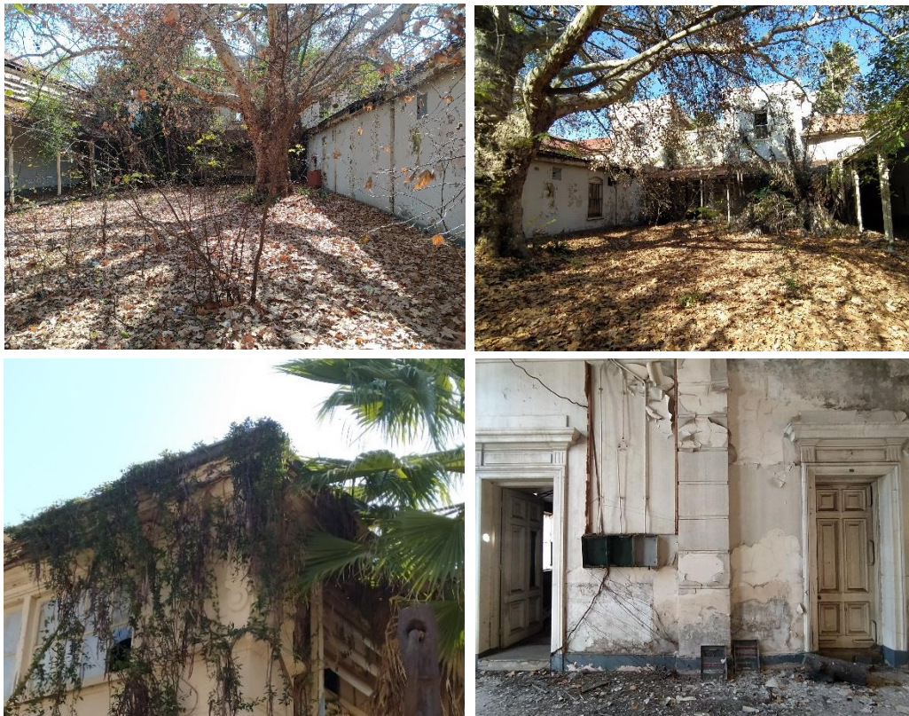
Figure 16. The present state of the Old Staatsmuseum. The building has been completely overtaken by an entropic layer of vegetation and ruination. (clockwise top left) the existing courtyard, looking north; courtyard looking south; a corner of the clerestories; inside the main entrance foyer (Author 2022)
