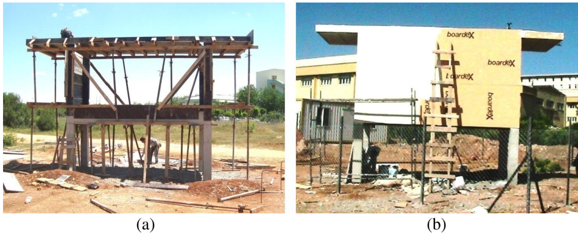
Figure 2.14: Abid et al. (2016) experimental box-girder segment: (a) formwork construction, (b) sealing with isolation boards.
