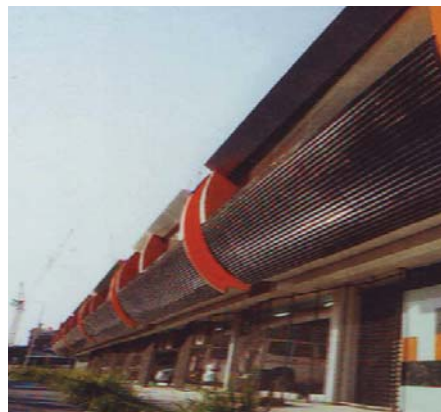
116. State Emergency Services Headquarters - Fractured Facade
