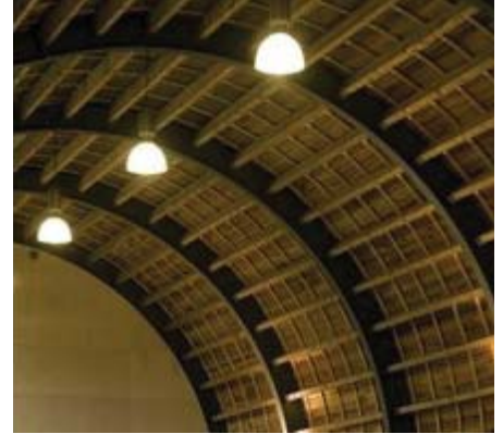
120. Sheep Stable - Lighting Detail
