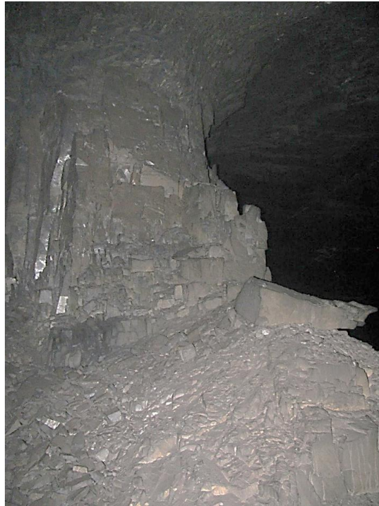
Figure 12-21. Side C of pillar N3_2 at Nchwaning III shaft illustrating the right-hand corner of the pillar as observed on the 18th of August 2021.
