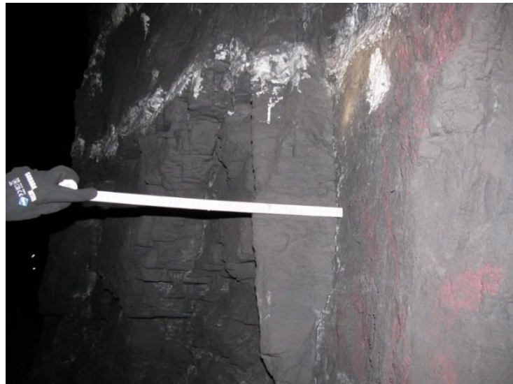
Figure 3-26. The vertical joint spacing is observed on side C of the pillar with a spacing of approximately 20 cm.
