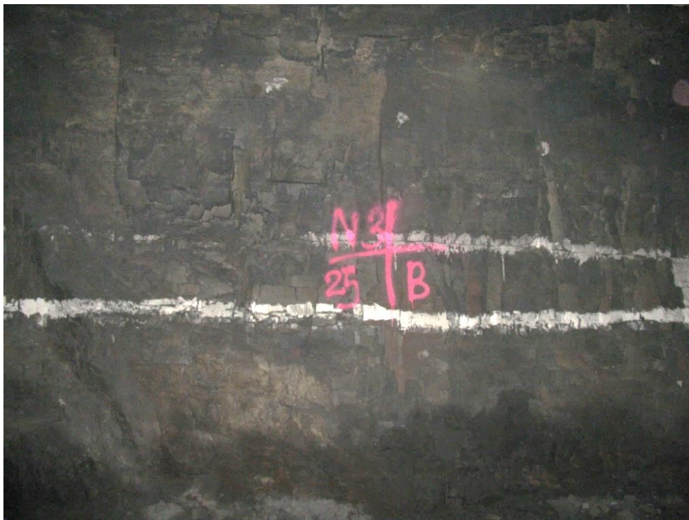
Figure 12-60. Side B of pillar N3_25 at Nchwaning III shaft as observed on the 6 th of May 2021.
