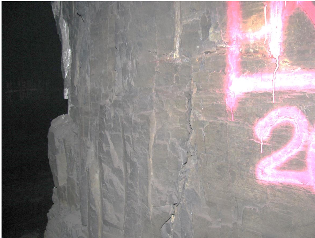
Figure 12-56. Side D of pillar N3_20 at Nchwane III shaft, illustrating the vertical joint opening on the side.
