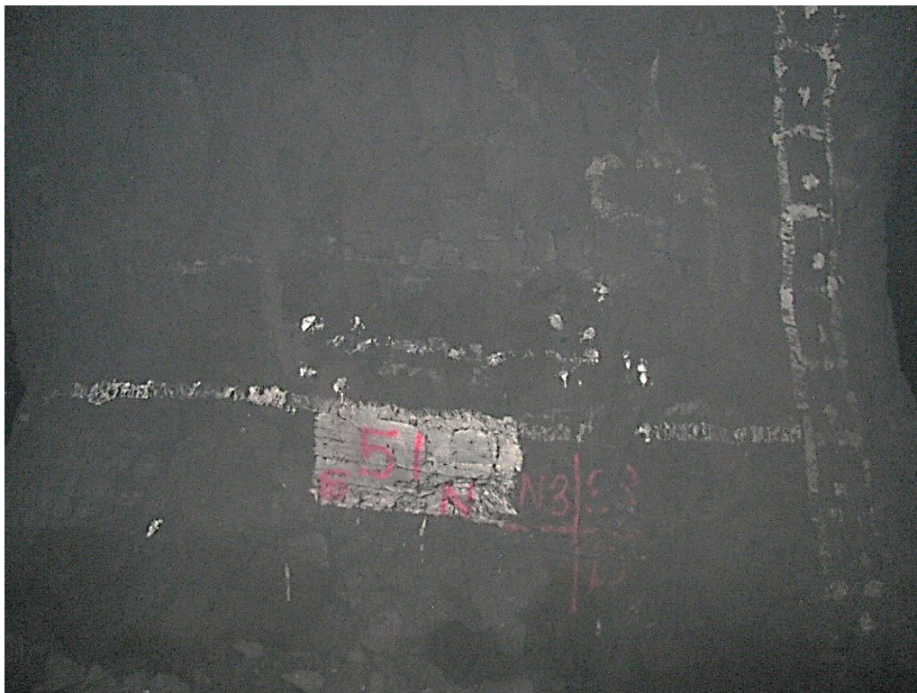
Figure 12-92. Side D of pillar N3_38 at Nchwaning III shaft as observed on the 18 th of August 2021.
