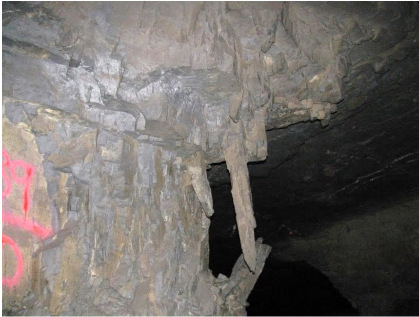
Figure 3-12. Extensive scaling of pillar N3_9. The scaling is facilitated by the intersecting horizontal and vertical joint sets.
