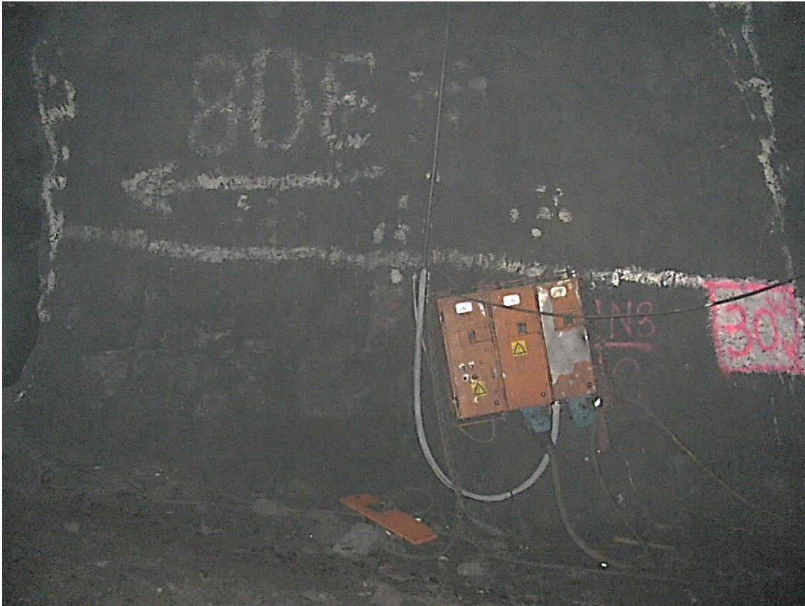
Figure 12-73. Side C of pillar N3_28 at Nchwane III shaft as observed on the 18th of August 2021.
