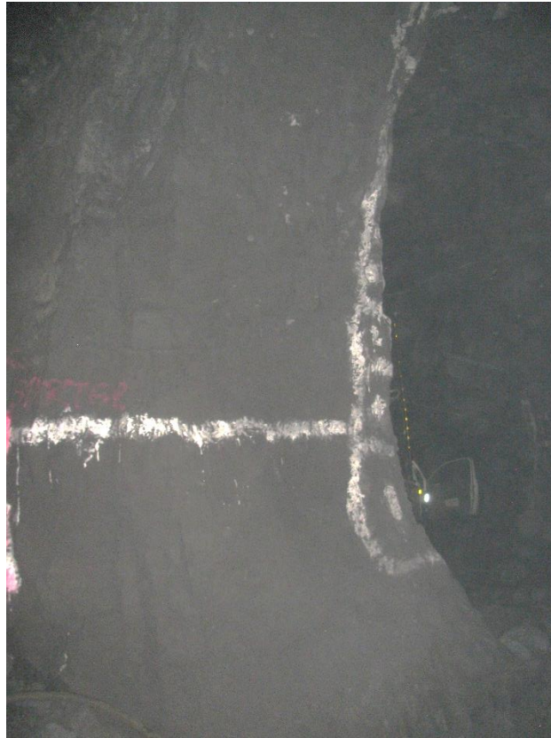
Figure 12-71. Side B of pillar N3_28 at Nchwaning III shaft, illustrating the left-hand side of the pillar as observed on the 18th of August 2021.
