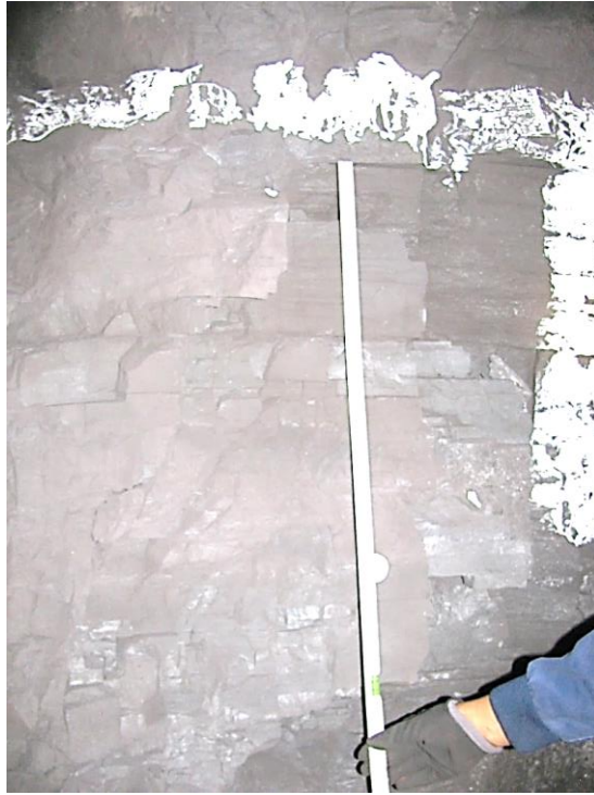
Figure 12-93. Side D of pillar N3_38 at Nchwaning III shaft, illustrating the horizontal joint spacing.
