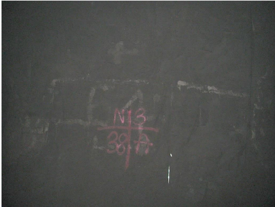
Figure 12-85. Side A of pillar N3_38 at Nchwaning III shaft as observed on the 18 th of May 2021.
