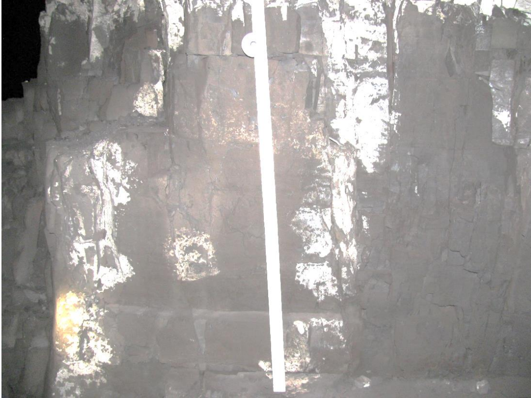
Figure 12-63. Side B of pillar N3_25 at Nchwaning III shaft, illustrating the horizontal joint spacing.
