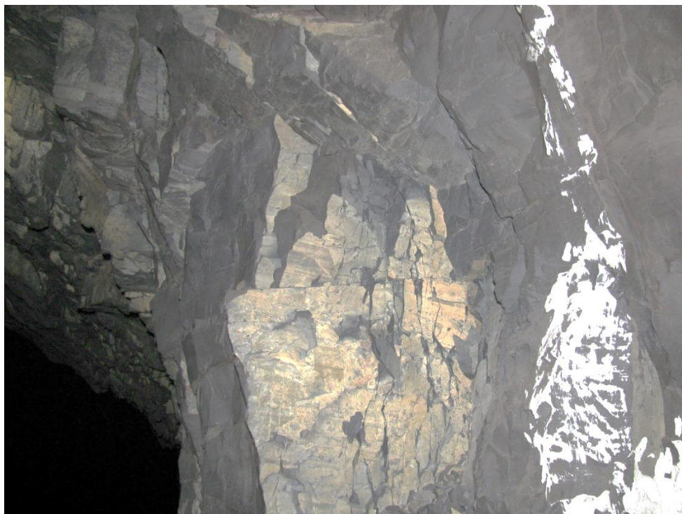
Figure 12-38. Side A of pillar N3_15 at Nchwaning III shaft, illustrating slight weathering on the corner.
