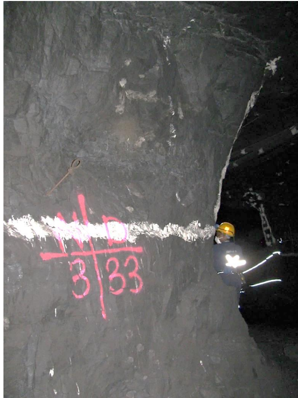
Figure 12-83. Side D of pillar N3_33 at Nchwaneing III shaft, illustrating the right-hand corner of the pillar as observed on the 17 th of May 2021.
