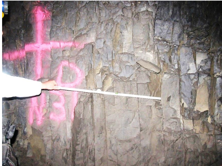
Figure 11-3. Joint spacing on Side D (right corner) of the pillar indicates a vertical joint spacing of approximately 10 cm.
