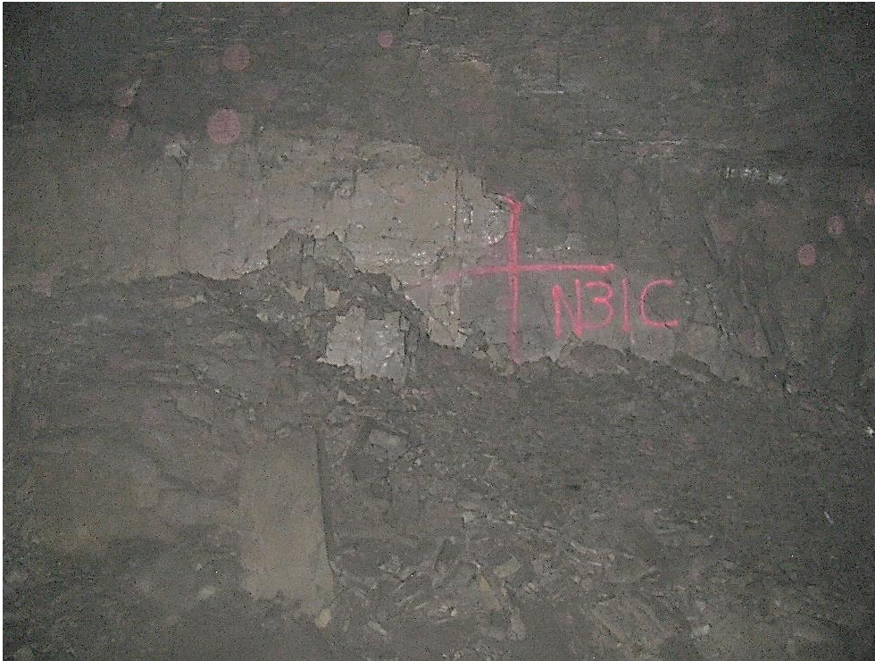
Figure 12-7. Side C of pillar N3_1 at Nchwaning III shaft as observed on the 4 th of May 2021.
