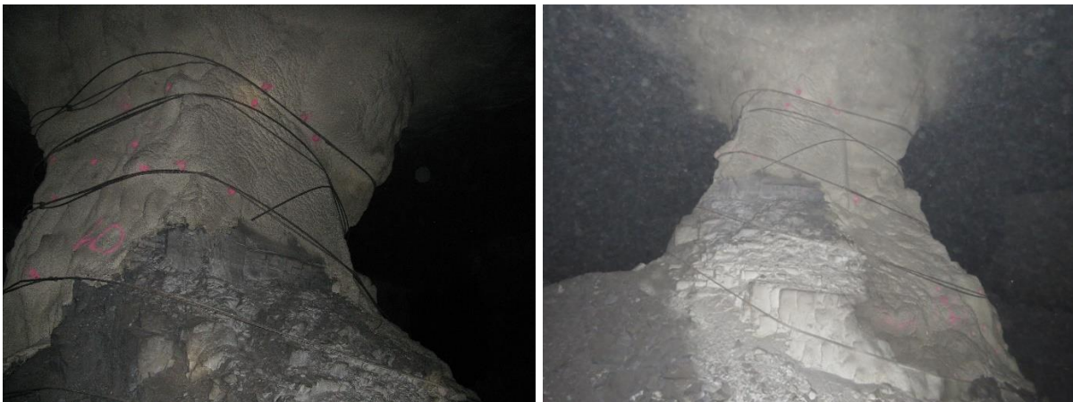
Figure 5-17. Condition of pillar P60.
