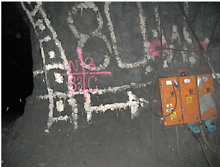
Figure 12-80. Side C of pillar N3_33 at Nchwaning III shaft as observed on the 17 th of May 2021.
