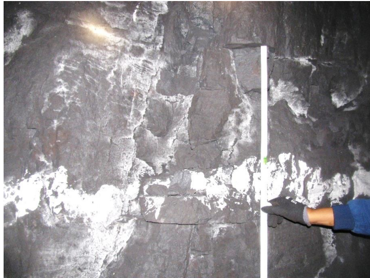
Figure 3-25. Side A of the pillar illustrates the horizontal joints with an approximate spacing of 50 cm.
