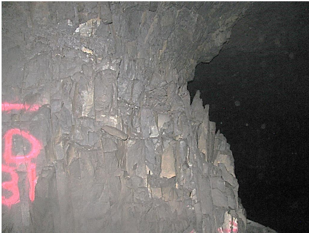
Figure 12-10. Side D of pillar N3_1 at Nchwaning III shaft illustrating the vertical joints on the right-hand corner of the pillar.
