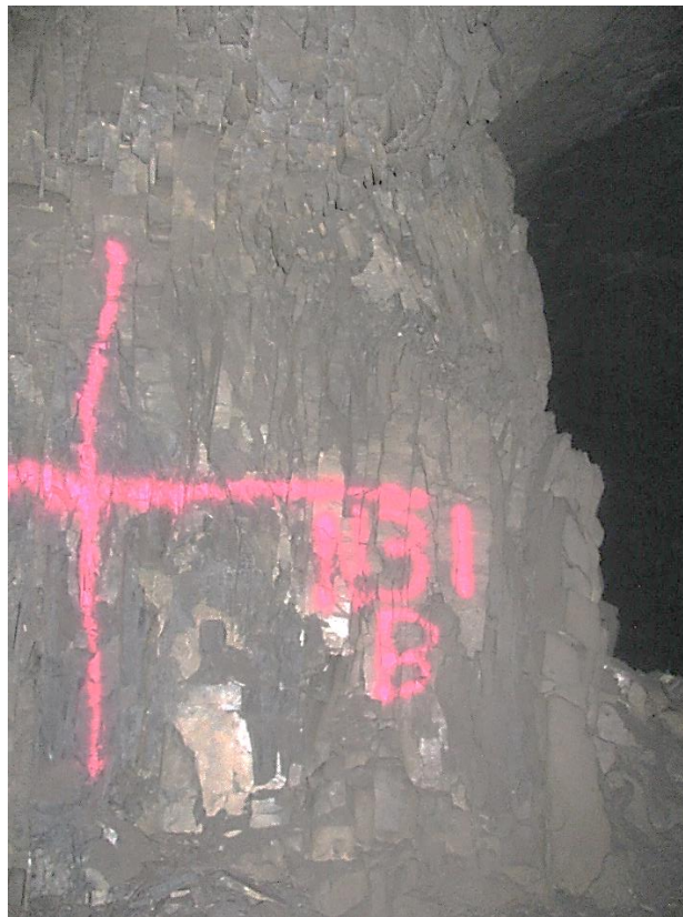
Figure 12-6. Side B of pillar N3_1 at Nchwaning III shaft illustrating buckling of the corner as observed on the 18th of August 2021. No time-dependent scaling took place over this period.
