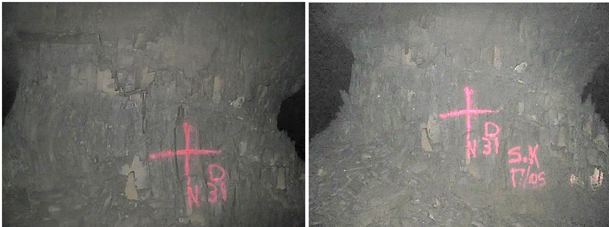
Figure 3-7. Almost no scaling was recorded for most of the pillars over a three-month monitoring period. As an example, this is pillar N3_1 at Nchwaning III Shaft. The photograph on the left was taken on 6 May 2021 and the photograph on the right on 18 August 2021.
