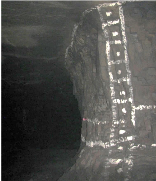
Figure 12-65. Side D of pillar N3_25 at Nchwaning III shaft, illustrating the left-hand corner of the pillar and no additional scaling of the corners was observed.
