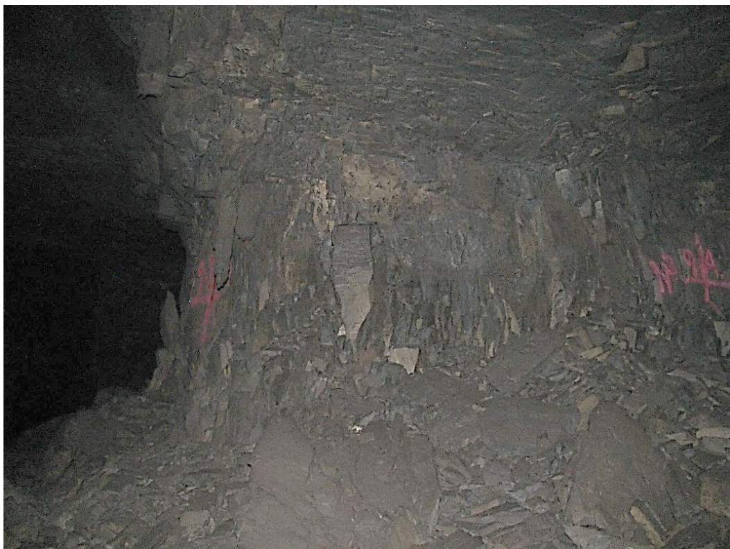
Figure 12-26. Side A of pillar N3_9 at Nchwaneing III shaft, illustrating the vertical joint sets and the size of the block that are scaling off the pillar on the left-hand side.
