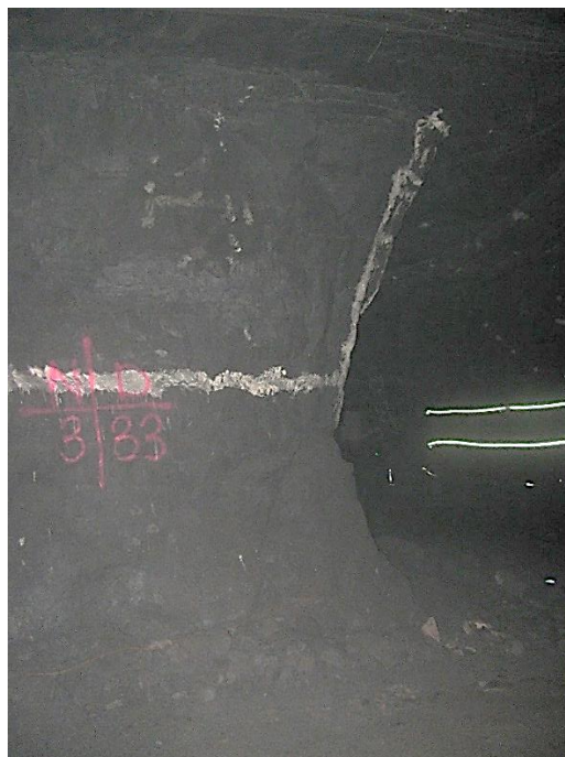
Figure 12-84. Side D of pillar N3_33 at Nchwaneing III shaft, illustrating the right-hand corner of the pillar as observed on the 18 th of August 2021.
