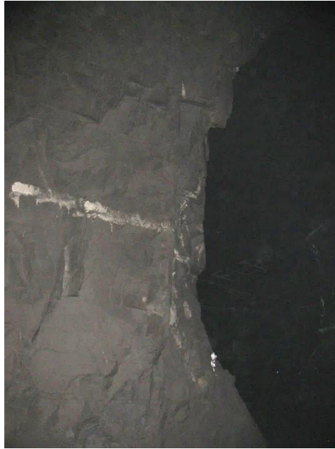
Figure 3-29. The corner of the pillar as viewed from side A. An hourglass shape was observed.
