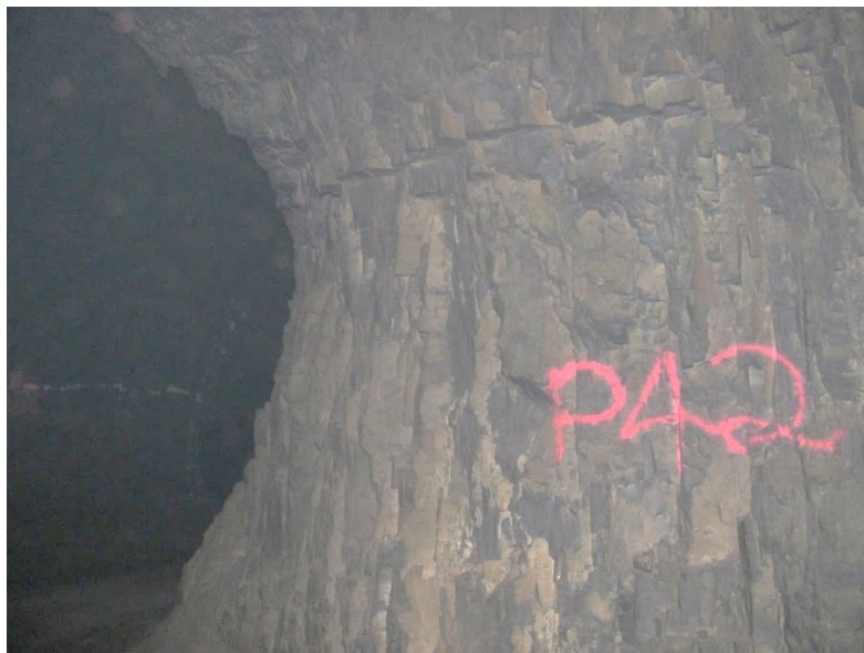
Figure 12-46. Side A of pillar N3_20 at Nchwanning III shaft, illustrating the left-hand corner of the pillar as observed on the 6 th of May 2021.
