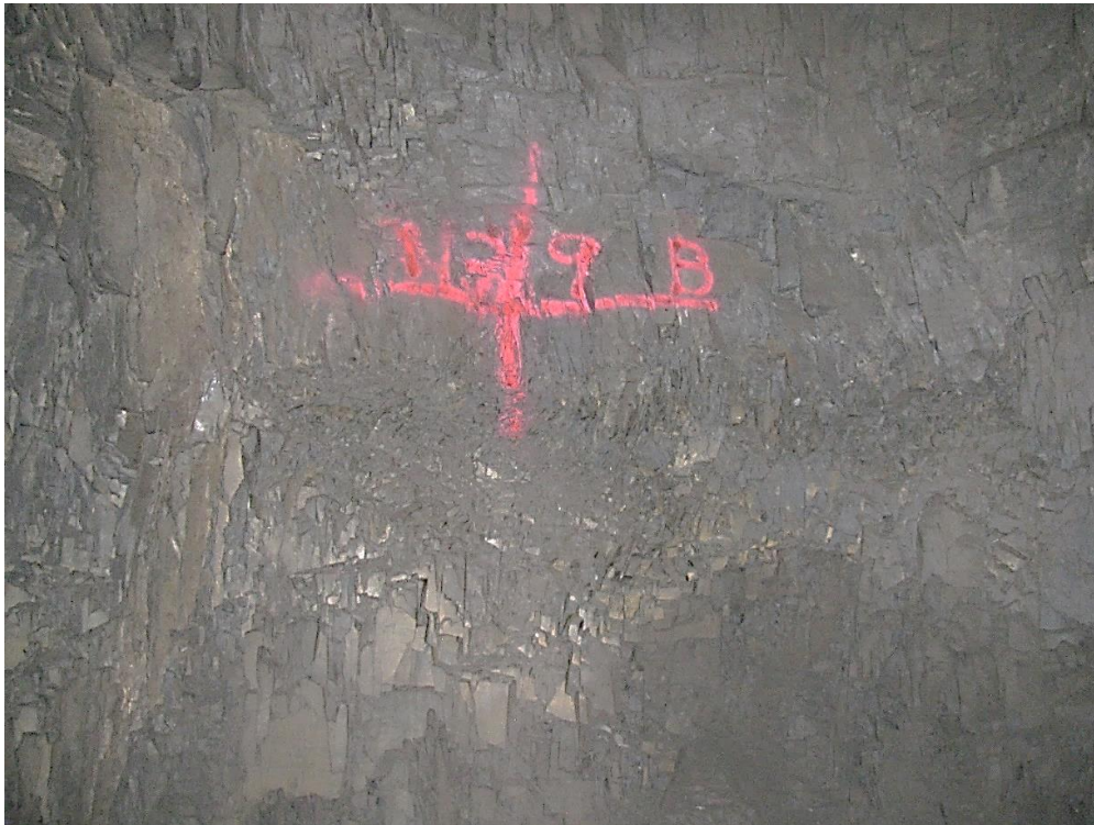
Figure 12-27. Side B of pillar N3_9 at Nchwaning III shaft as observed on the 4 th of May 2021.
