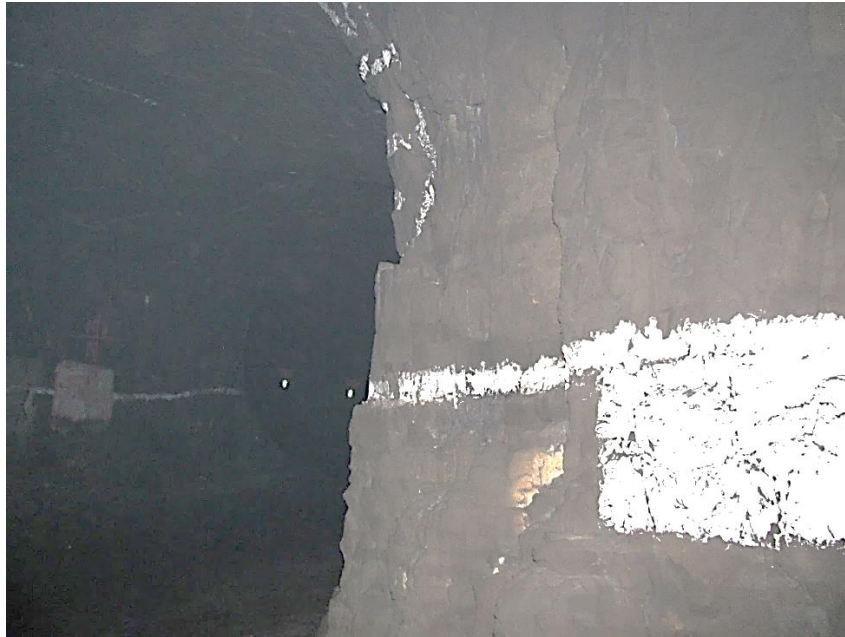
Figure 12-45. Side D of pillar N3_15 at Nchwanning III shaft, illustrating the condition of the left-hand corner of the pillar.
