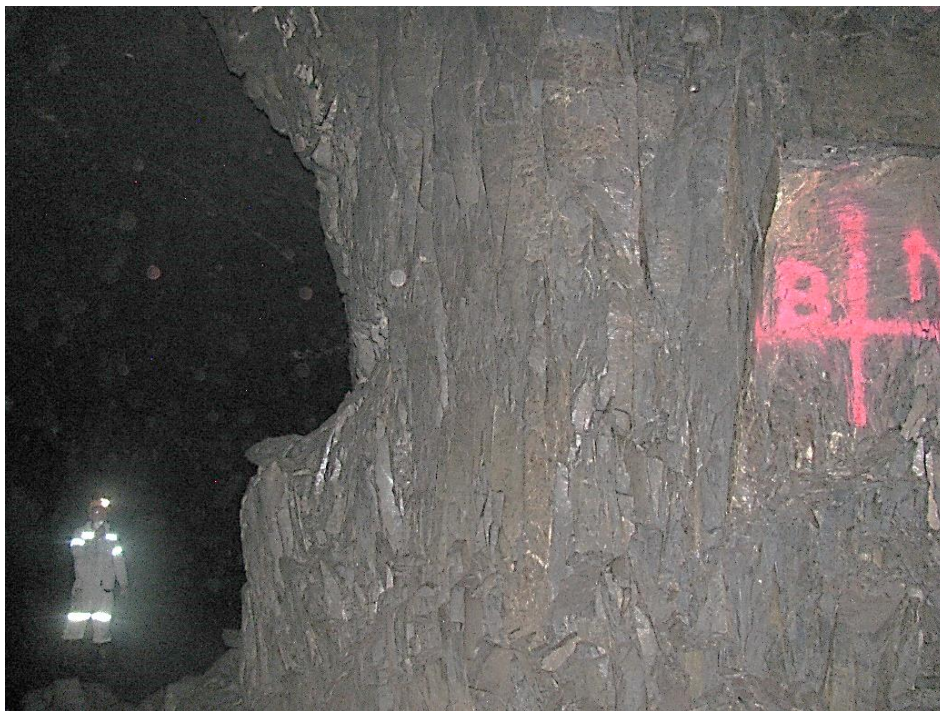
Figure 12-16. Side B of pillar N3_2 at Nchwaning III shaft illustrating the vertical joint sets on the left-hand corner of the pillar.
