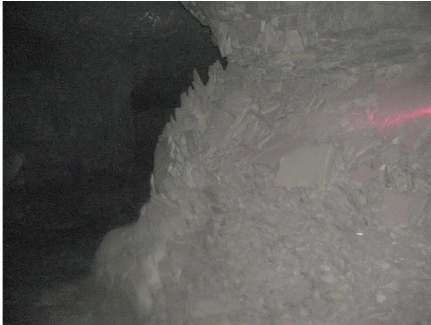
Figure 12-3. The left corner of side A of pillar N3_1 at Nchwaneing III shaft as observed on the 4 th of May 2021.
