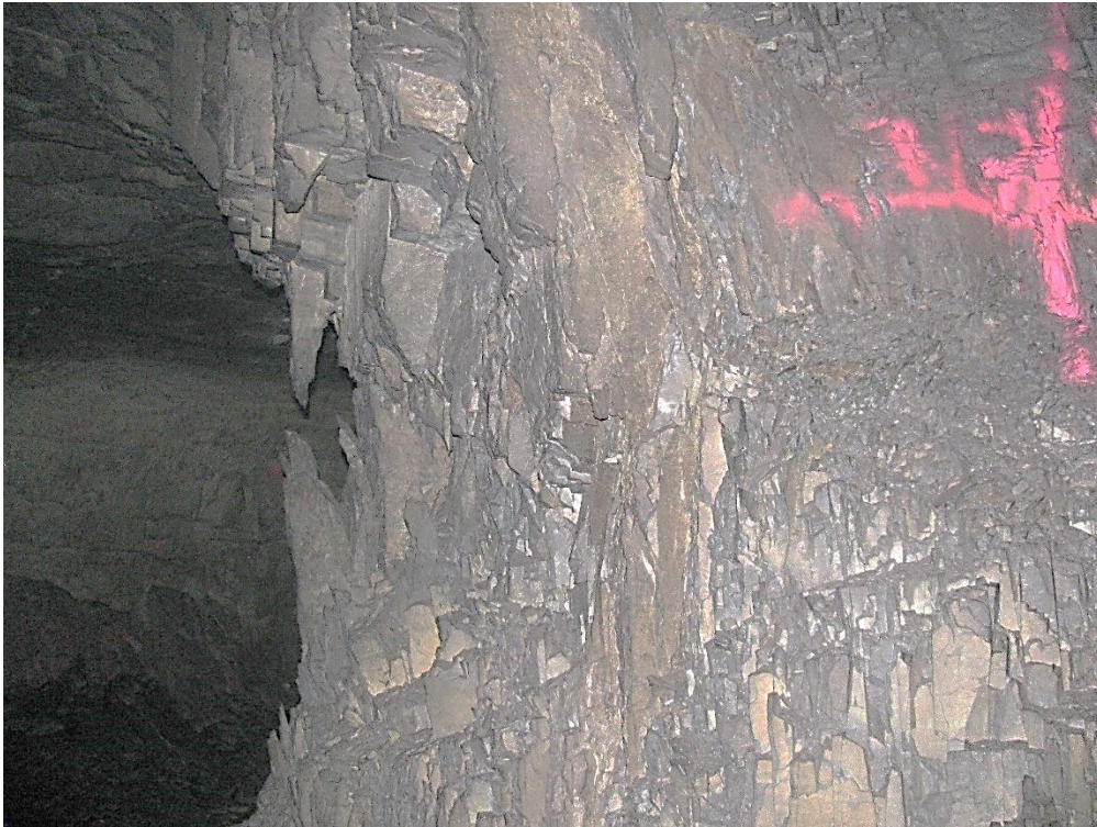
Figure 12-31. Side B of pillar N3_9 at Nchwaning III shaft, illustrating the vertical joint sets on the left-hand corner as observed on the 18th of August 2021.
