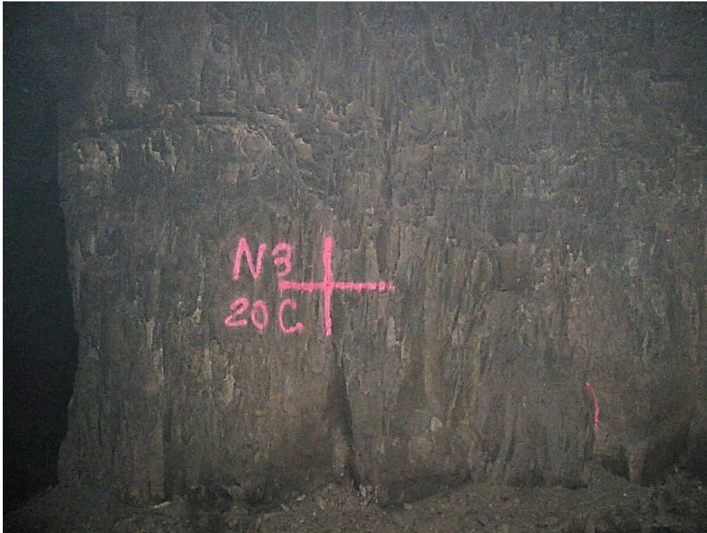
Figure 12-51. Side C of pillar N3_20 at Nchwane III shaft as observed on the 6 th of May 2021.
