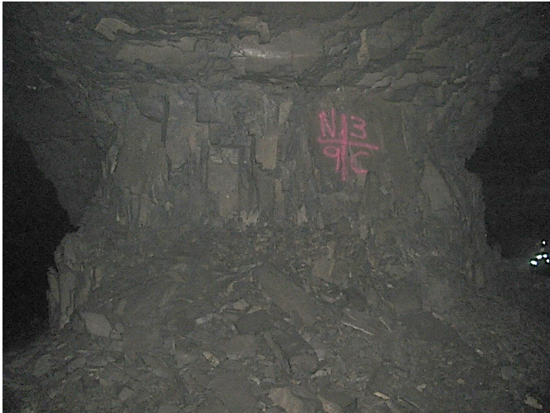
Figure 12-33. Side C of pillar N3_9 at Nchwaning III shaft as observed on the 18th of August 2021.
