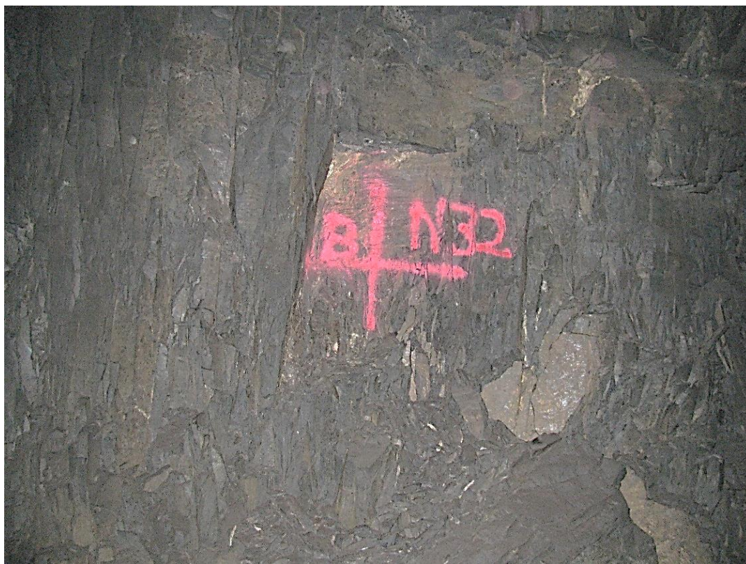
Figure 12-14. Side B of pillar N3_2 at Nchwane III shaft as observed on the 4 th of May 2021.
