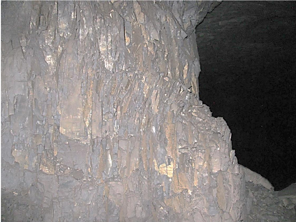
Figure 12-29. Side B of pillar N3_9 at Nchwaning III shaft, illustrating the vertical joint sets as observed on the 4 th of May 2021.
