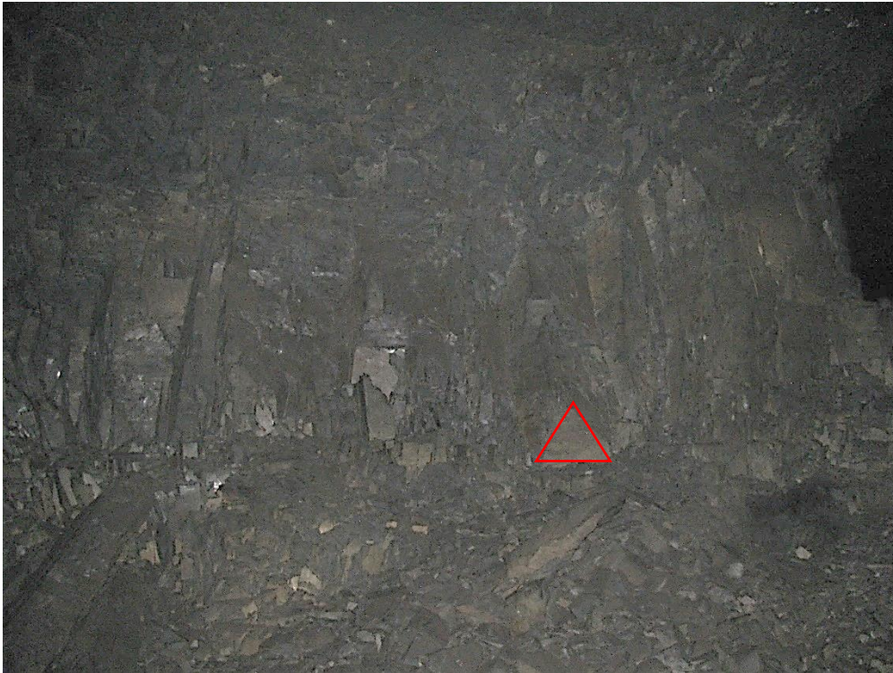
Figure 12-19. Side C of pillar N3_2 at Nchwaneing III shaft, the red triangle was used as a reference point to measure the scaling distance as the pillar was too dangerous to mark. This photograph was taken on the 18th of August 2021.
