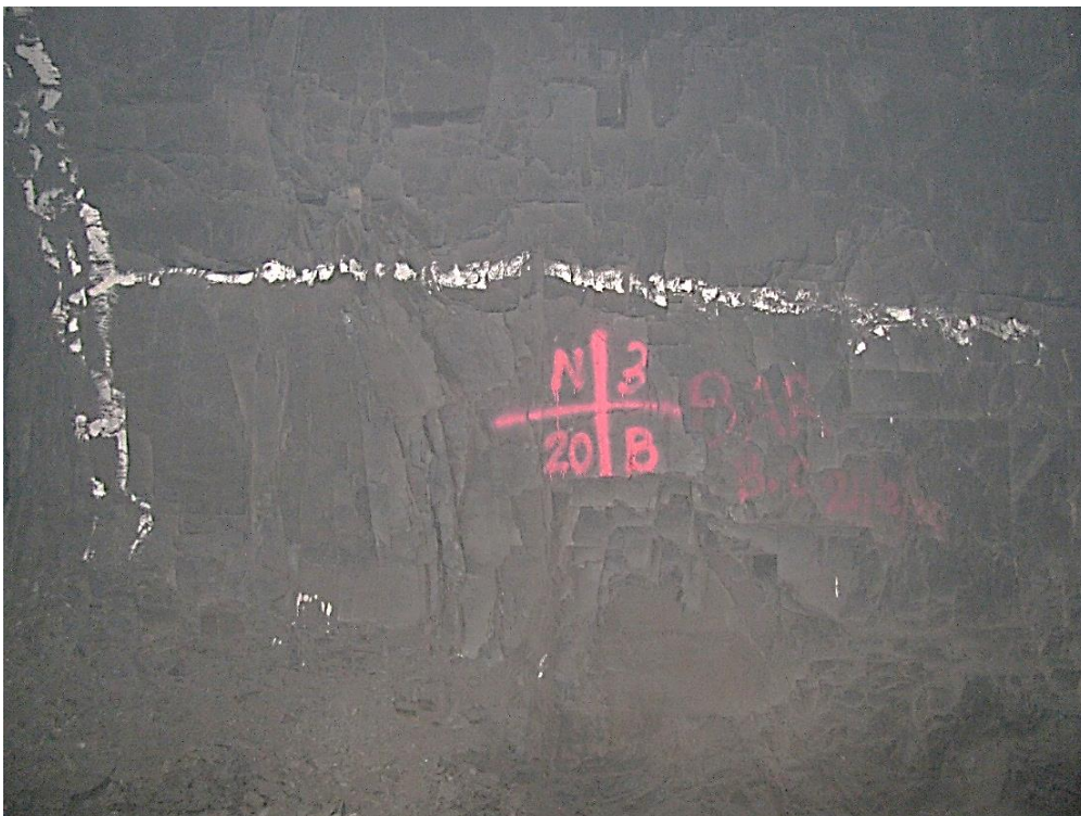
Figure 12-48. Side B of pillar N3_20 at Nchwaning III shaft as observed on the 6 th of May 2021.
