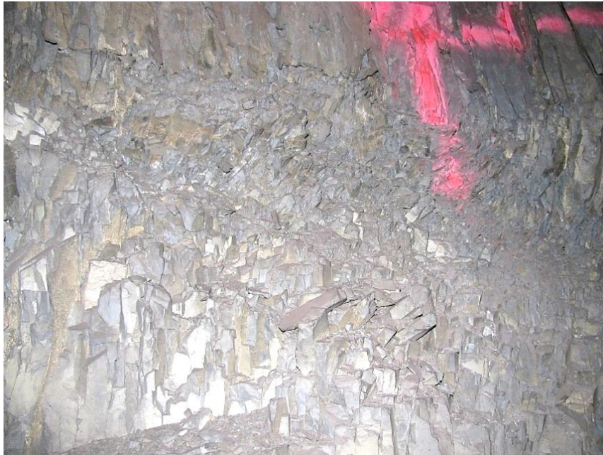
Figure 3-11. Side B of the pillar illustrates the closely spaced joint sets. This creates extensive scaling on the sides of the pillar.
