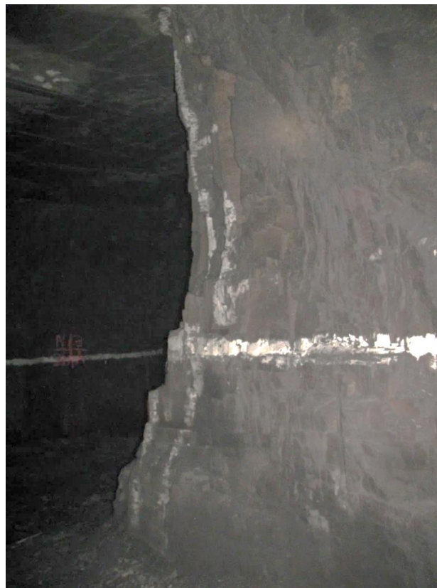
Figure 12-62. Side B of pillar N3_25 at Nchwaning III shaft, illustrating the hourglass shape on the left-hand corner of the pillar.
