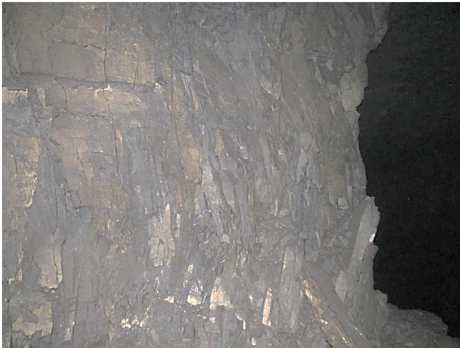
Figure 12-24. Side D of pillar N3_2 at Nchwane III shaft, illustrating the vertical joint sets on the right-hand corner of the pillar as observed on the 18 th of August 2021.
