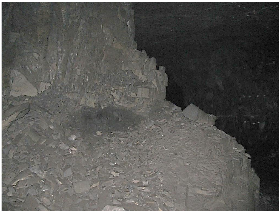
Figure 12-20. Side C of pillar N3_2 at Nchwaneing III shaft illustrating the right-hand corner of the pillar as observed on the 4 th of May 2021.
