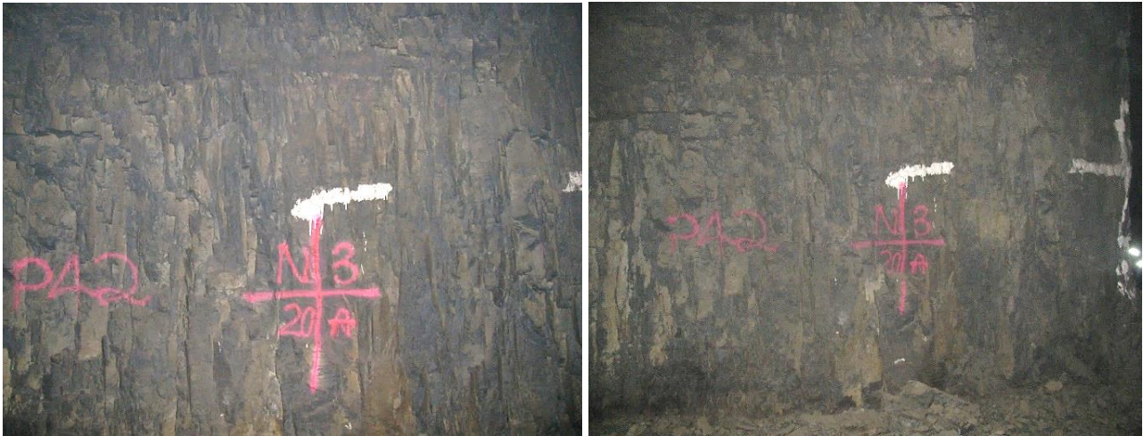
Figure 3-18. Side A of pillar N3_20 at Nchwaning III shaft as photographed on the 6 May 2021 (left) and on 18 August 2021 (right).
