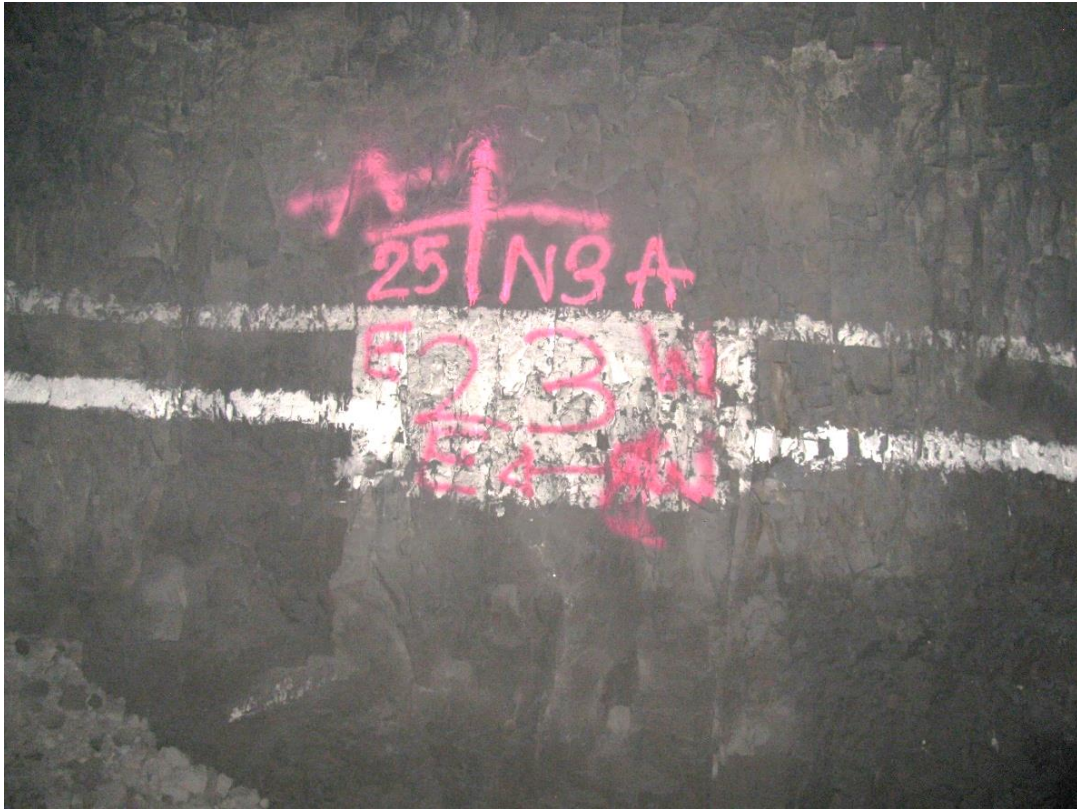
Figure 12-57. Side A of pillar N3_25 at Nchwaning III shaft as observed on the 6 th of May 2021.
