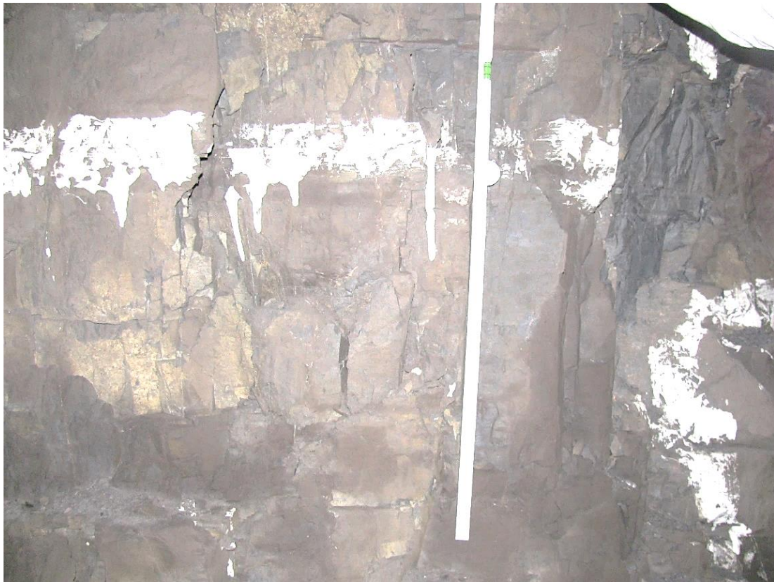
Figure 12-40. Side B of pillar N3_15 at Nchwaneing III shaft, illustrating the horizontal joint spacing.
