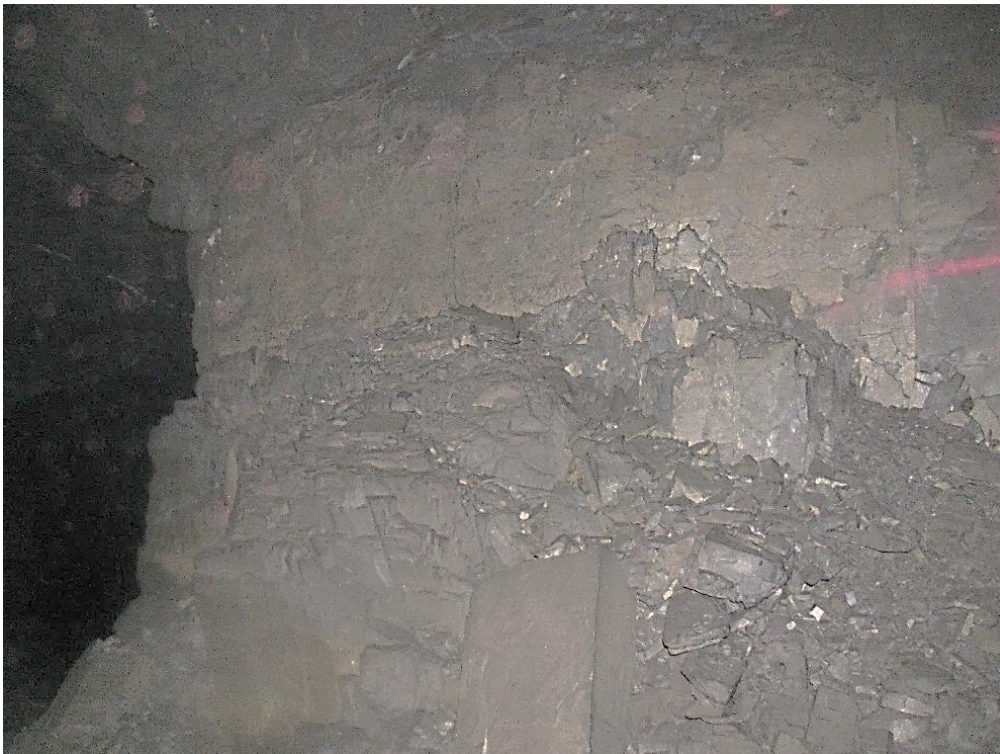
Figure 12-8. Side C of pillar N3_1 at Nchwaning III shaft illustrating the scaling that has taken place since the pillar was cut.
