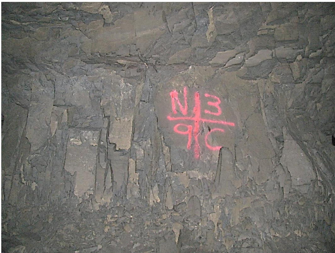
Figure 12-32. Side C of pillar N3_9 at Nchwaning III shaft as observed on the 4 th of May 2021.
