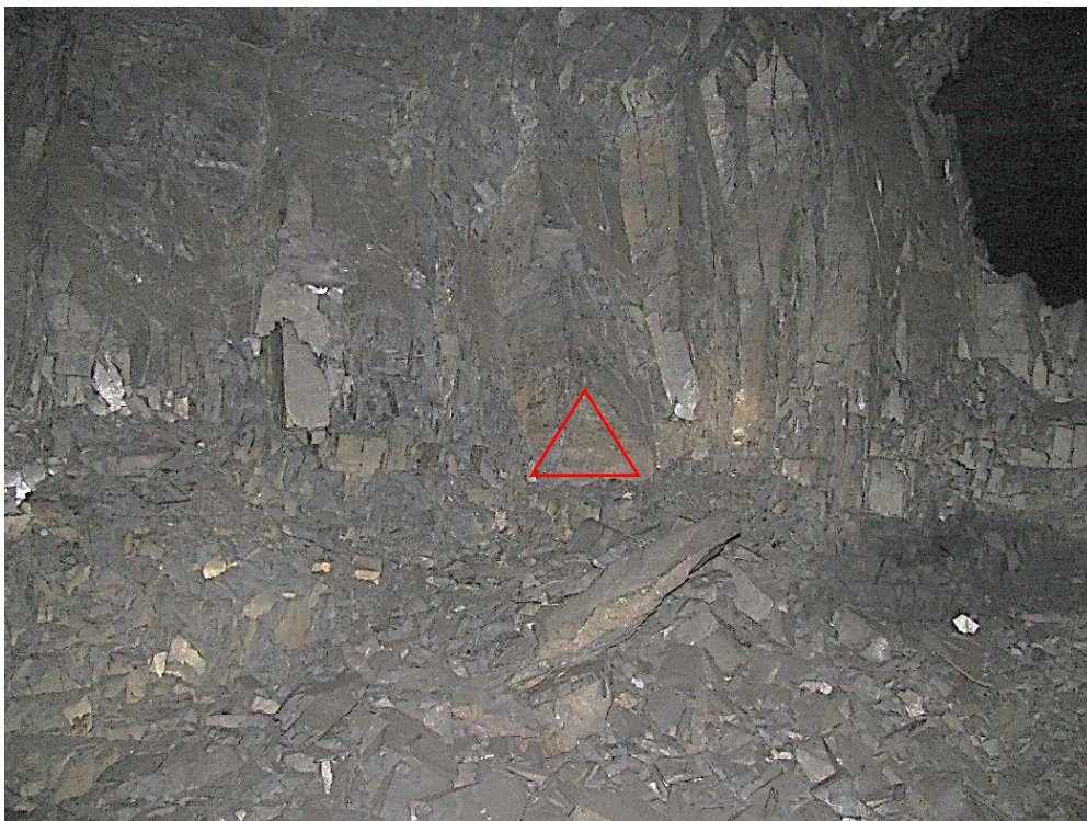
Figure 12-18. Side C of pillar N3_2 at Nchwane III shaft as observed on the 4 th of May 2021, the red triangle was used as a reference point to measure the scaling distance as the pillar was too dangerous to mark
