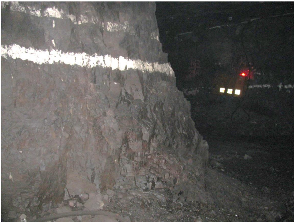
Figure 12-58. Side A of pillar N3_25 at Nchwaning III shaft, illustrating the condition of the right-hand corner of the pillar.
