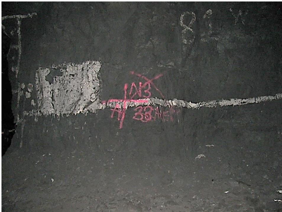
Figure 12-76. Side A of pillar N3_33 at Nchwaning III shaft as observed on the 17 th of May 2021.
