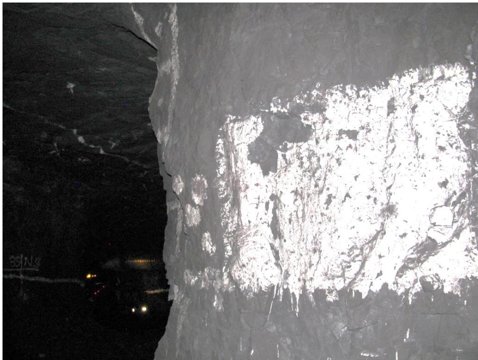
Figure 12-78. Side A of pillar N3_33 at Nchwaning III shaft, illustrating the left-hand corner of the pillar still in very good condition.
