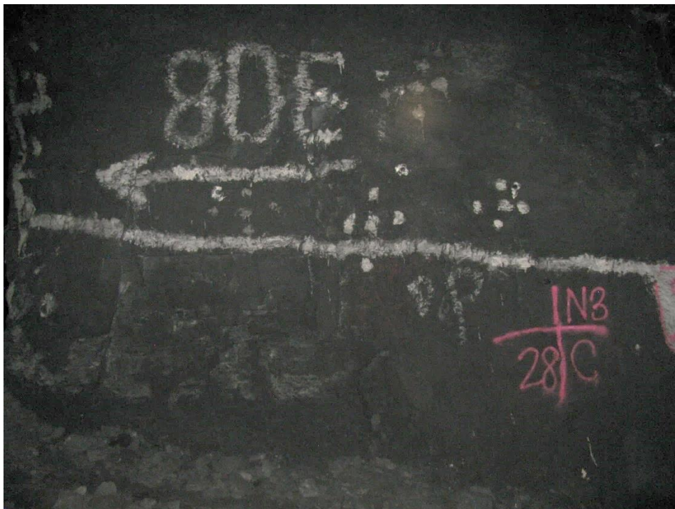
Figure 12-72. Side C of pillar N3_28 at Nchwaning III shaft as observed on the 17 th of May 2021.
