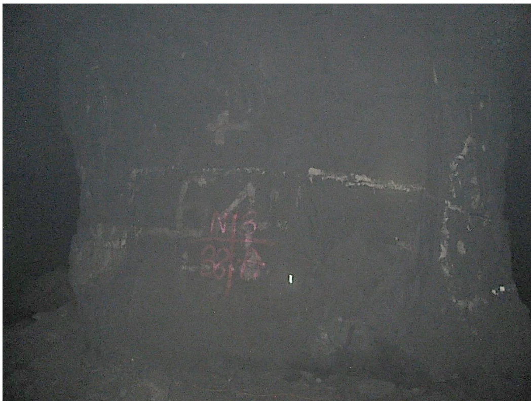
Figure 12-86. Side A of pillar N3_38 at Nchwaning III shaft as observed on the 18 th of August 2021.
