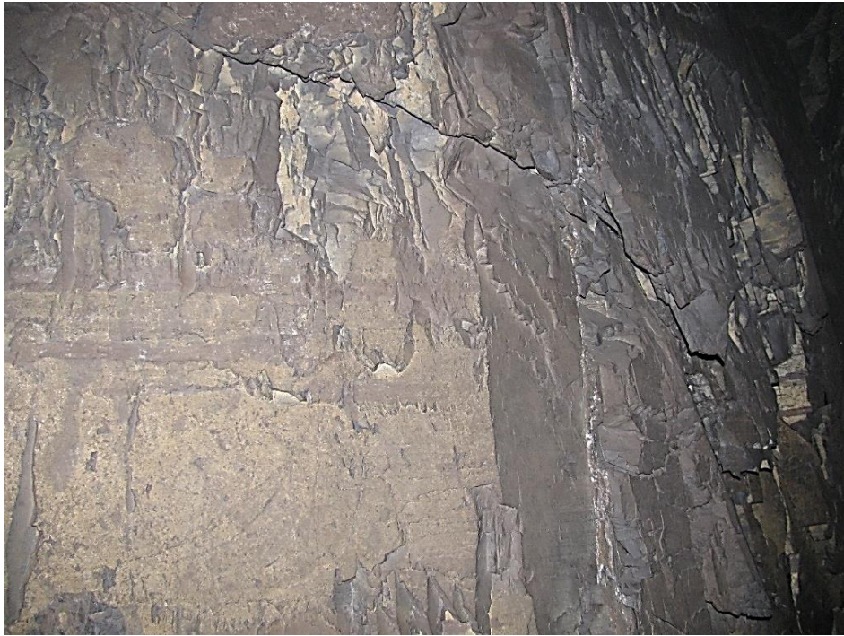
Figure 12-43. Side C of pillar N3_15 at Nchwane III shaft, illustrating the random joint terminating on Side C.
