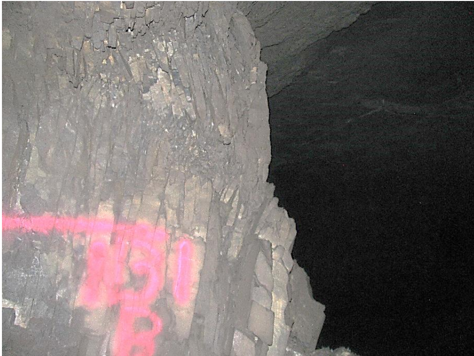
Figure 12-5. Side B of pillar N3_1 at Nchwaning III shaft illustrating buckling of the corner as observed on the 4 th of May 2021.
