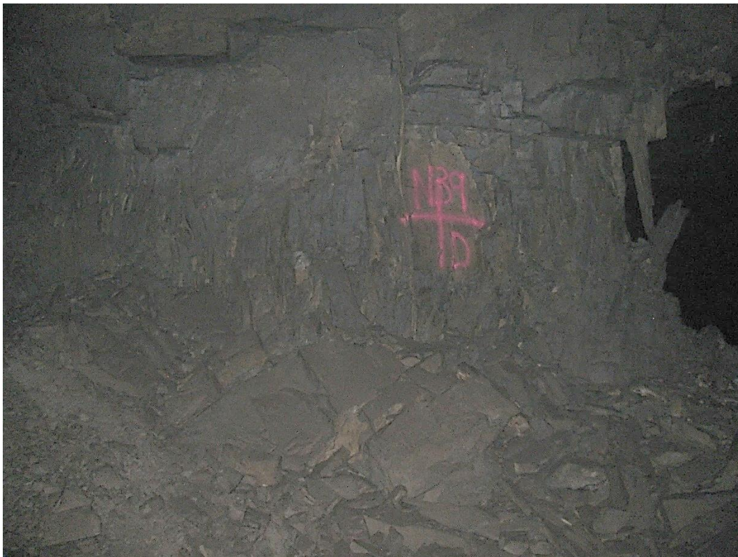
Figure 12-36. Side D of pillar N3_9 at Nchwaning III shaft as observed on the 18th of August 2021.
