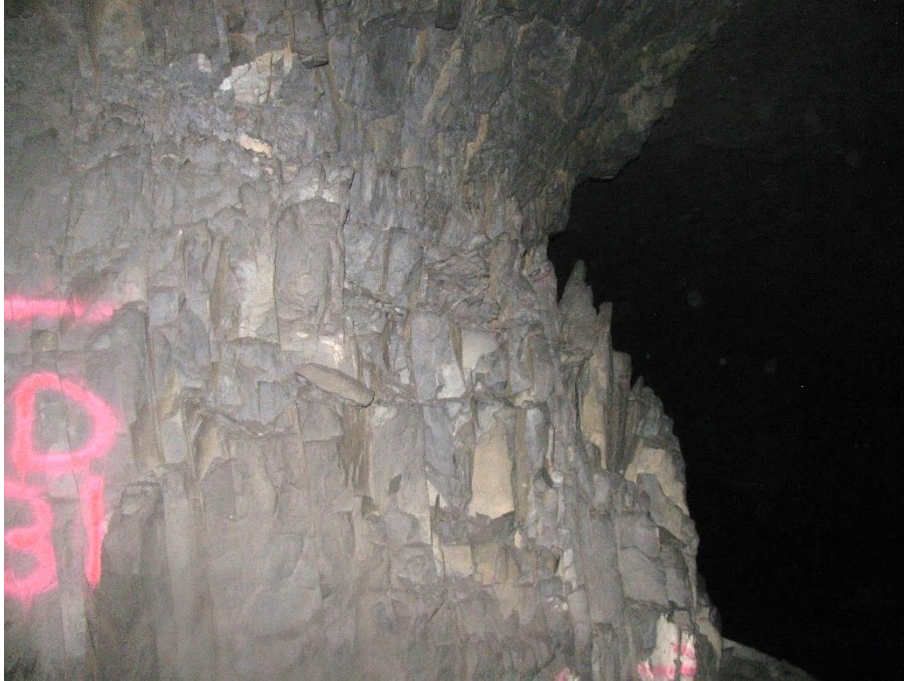
Figure 5-4. The condition of pillar N3_1 in Area 1 illustrating excessive scaling of the pillar.
