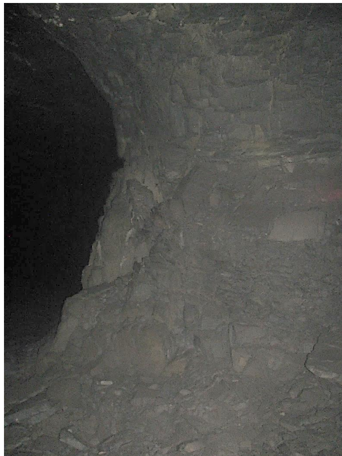
Figure 12-4. The left corner of side A of pillar N3_1 at Nchwaneing III shaft as observed on the 18th of August 2021.
