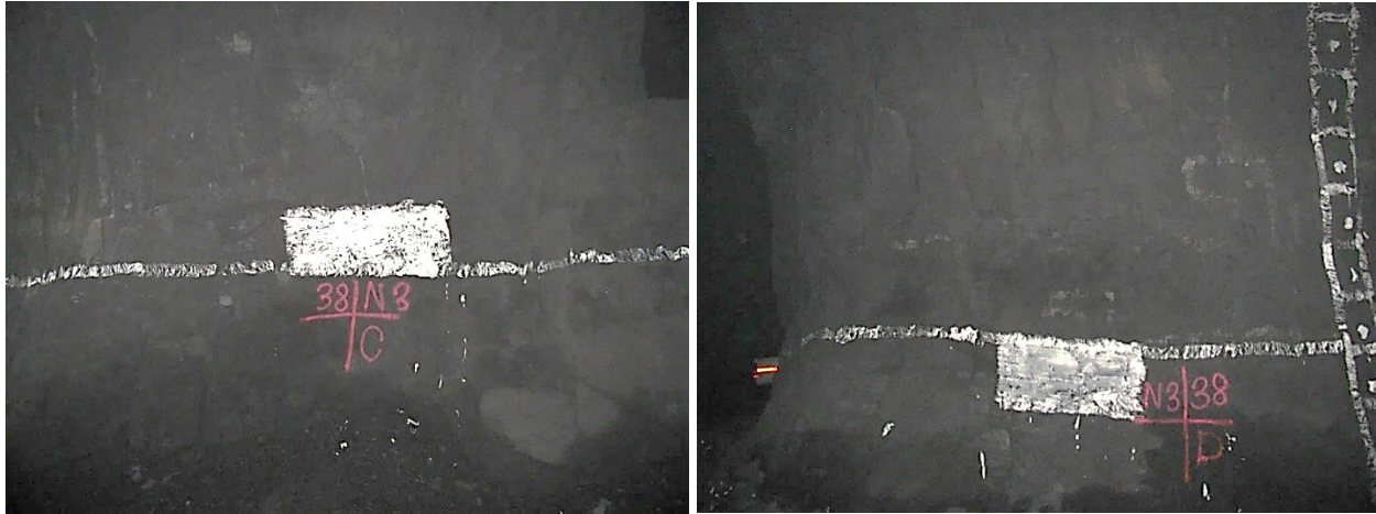
Figure 5-14. Two views of pillar N3_38 at Nchwaning III shaft illustrating the excellent condition of the pillar.
