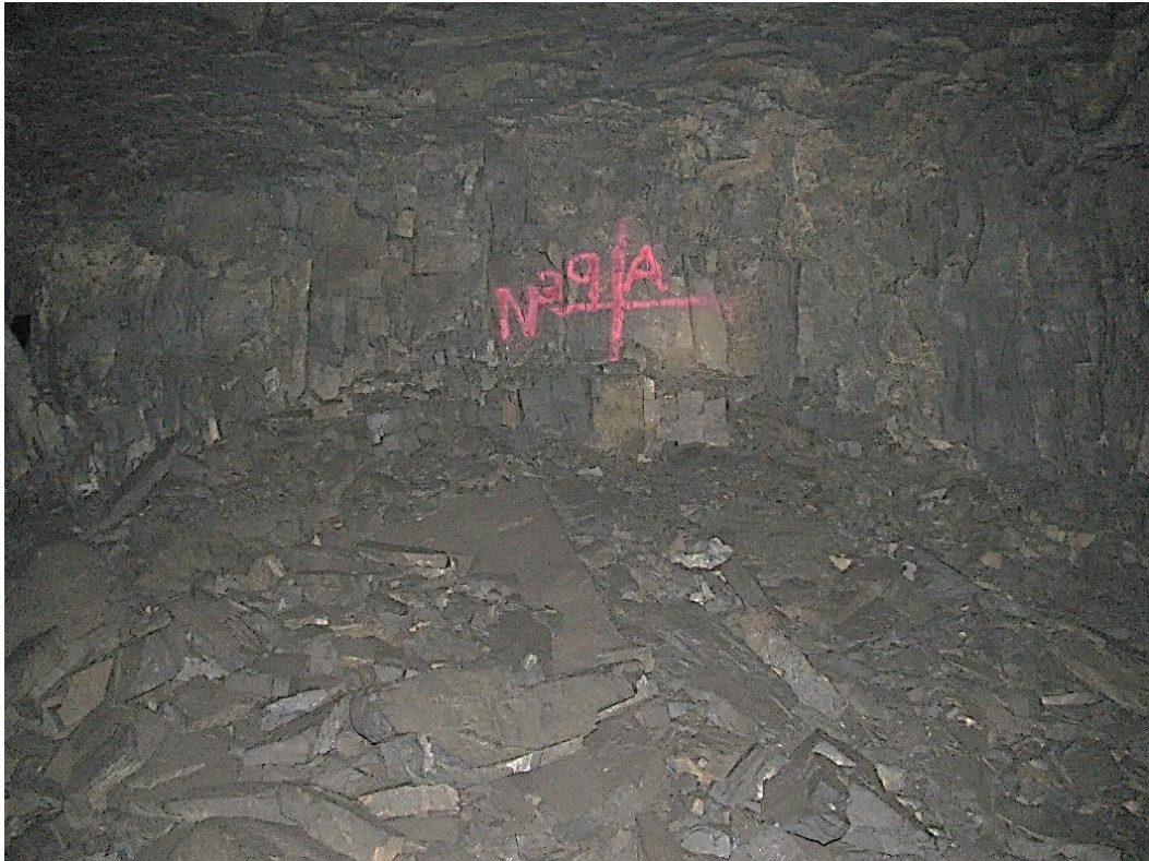
Figure 12-25. Side A of pillar N3_9 at Nchwaneing III shaft as observed on the 4 th of May 2021.
