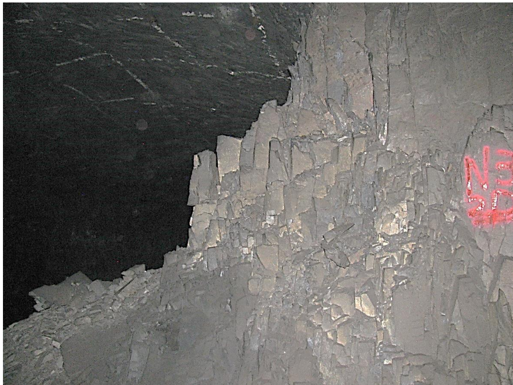
Figure 12-22. Side D of pillar N3_2 at Nchwaning III shaft, illustrating the vertical joint sets on the left-hand corner of the pillar.
