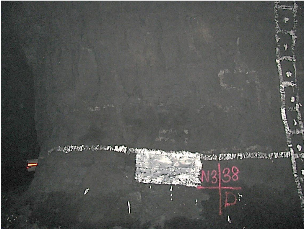
Figure 12-91. Side D of pillar N3_38 at Nchwaning III shaft as observed on the 18 th of May 2021.
