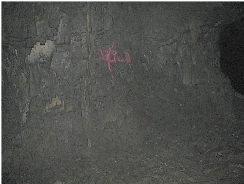
Figure 12-28. Side B of pillar N3_9 at Nchwaning III shaft as observed on the 18th of August 2021. A small amount of scaling took place.
