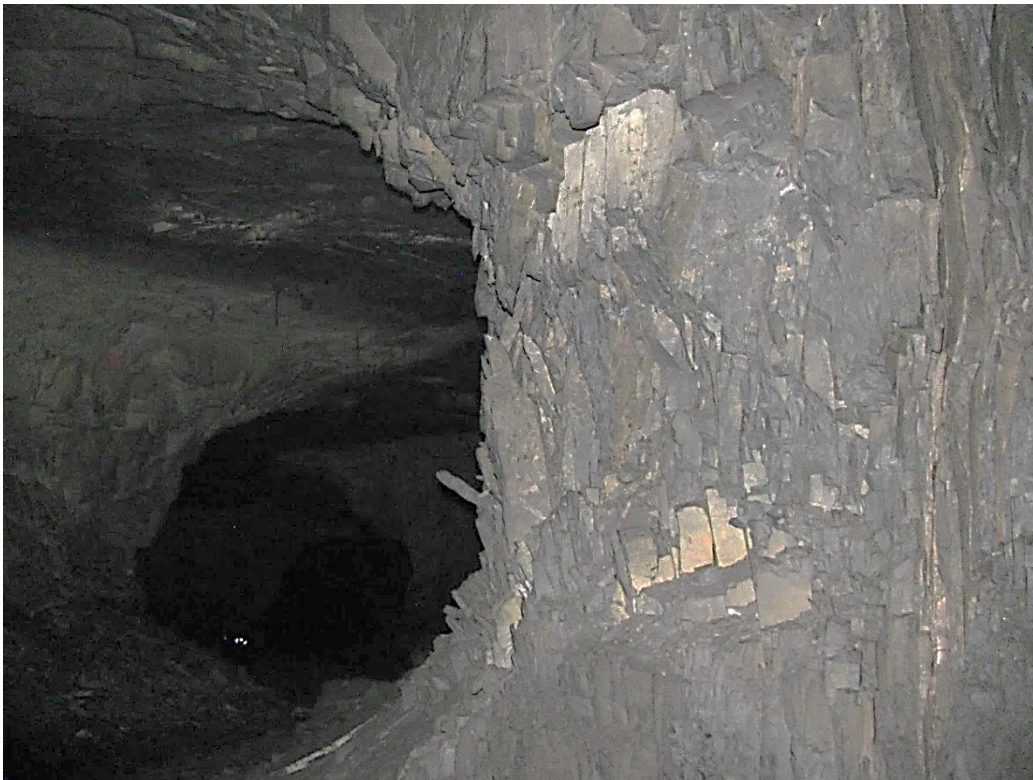
Figure 12-30. Side B of pillar N3_9 at Nchwaning III shaft, illustrating the vertical joint sets on the left-hand corner as observed on the 4 th of May 2021.
