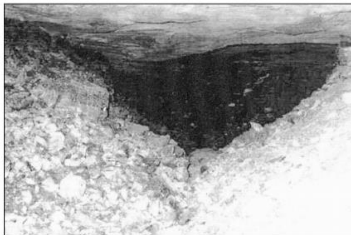
Figure 2-17. An area where scaling debris had built up to the height of the roof and pillar failure still continued (after Van der Merwe, 2003).
