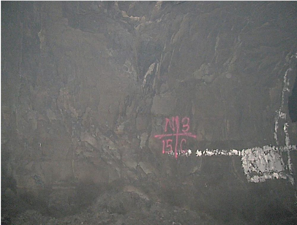
Figure 12-41. Side C of pillar N3_15 at Nchwane III shaft as observed on the 6 th of May 2021.
