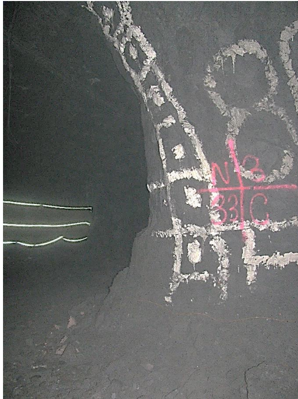
Figure 12-81. Side C of pillar N3_33 at Nchwaning III shaft as observed on the 18th of August 2021.
