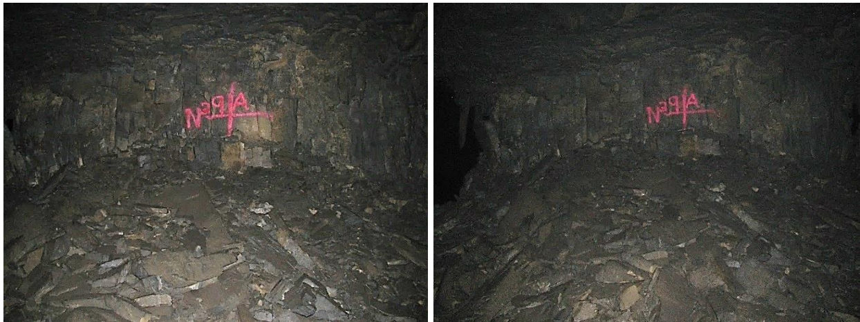
Figure 3-14. Side A of pillar N3_9 at Nchwaning III shaft observed on the 4 th of May (left) and on the 18 th of August 2021 (right).
