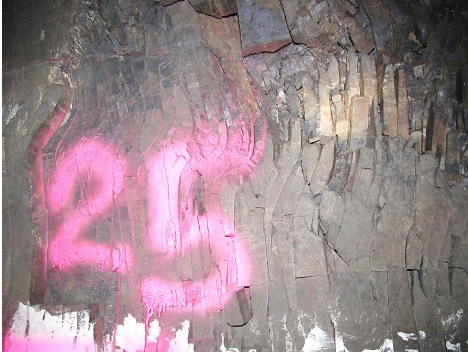
Figure 3-20. Complex jointing observed for pillar N3_25. Note the high density and curvature of the joints.
