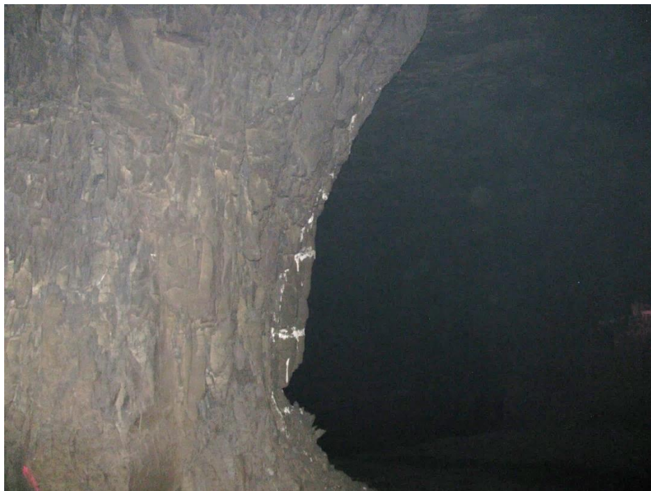
Figure 12-52. Side C of pillar N3_20 at Nchwane III shaft, illustrating the hourglass shape of the corner of the pillar.
