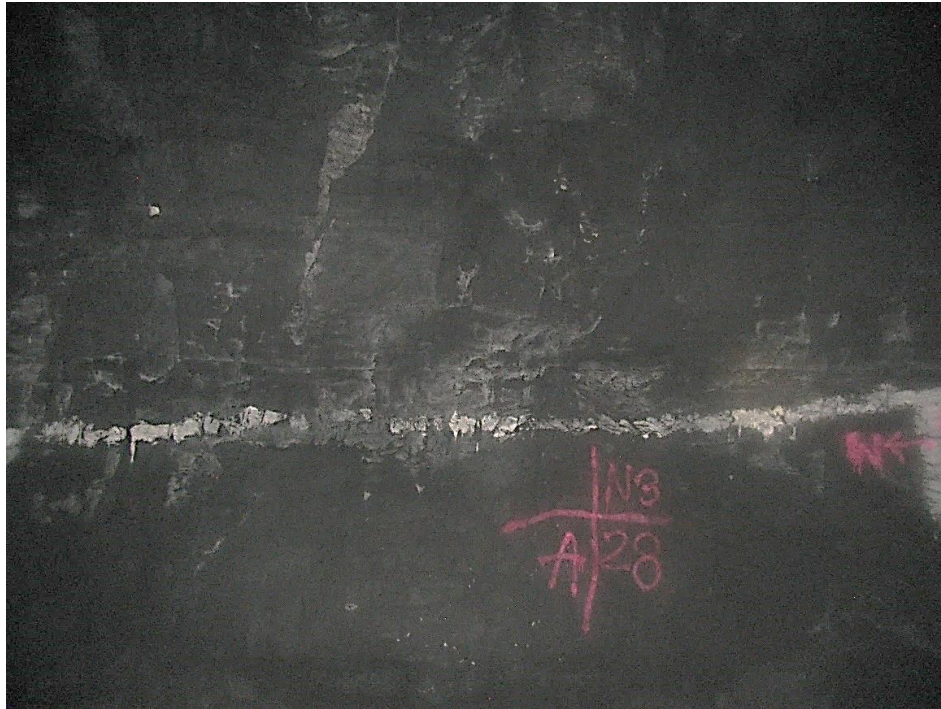
Figure 12-67. Side A of pillar N3_28 at Nchwane III shaft as observed on the 17 th of May 2021.
