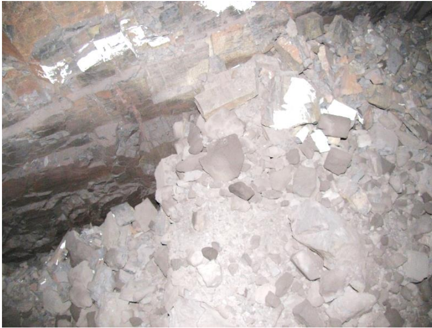
Figure 3-22. Small block sizes were found adjacent to pillar N3_25. These block sizes are controlled by the closely spaced joint sets.
