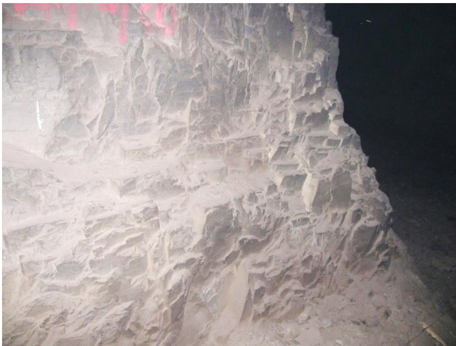
Figure 12-50. Side B of pillar N3_20 at Nchwaning III shaft, illustrating the right-hand corner of the pillar.
