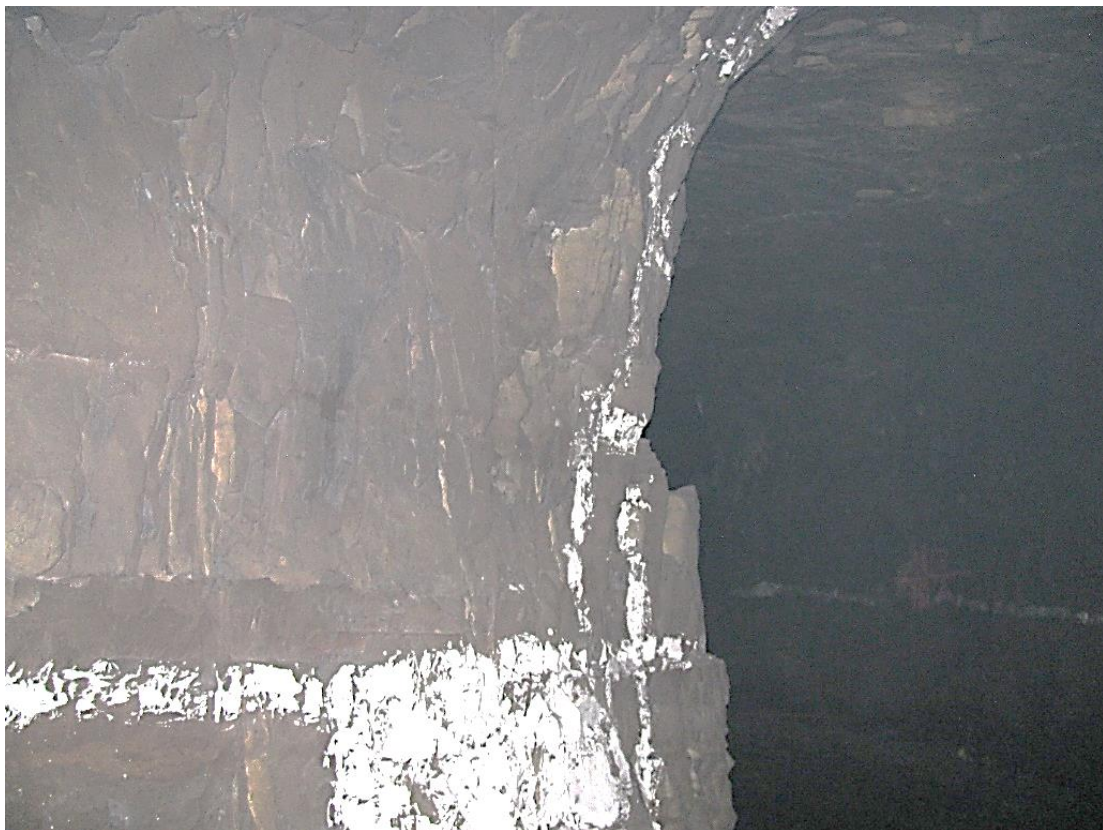
Figure 12-42. Side C of pillar N3_15 at Nchwane III shaft, illustrating the condition of the right-hand corner of the pillar.
