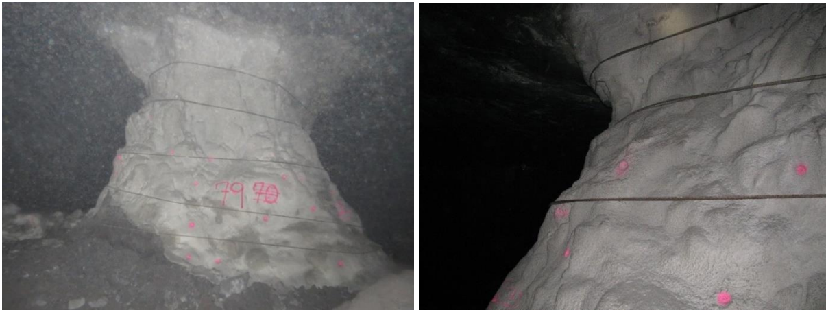
Figure 5-18. Condition of pillar P79.
