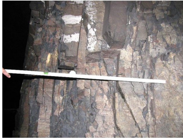
Figure 5-10. Extensive scaling of pillar N3_25.
