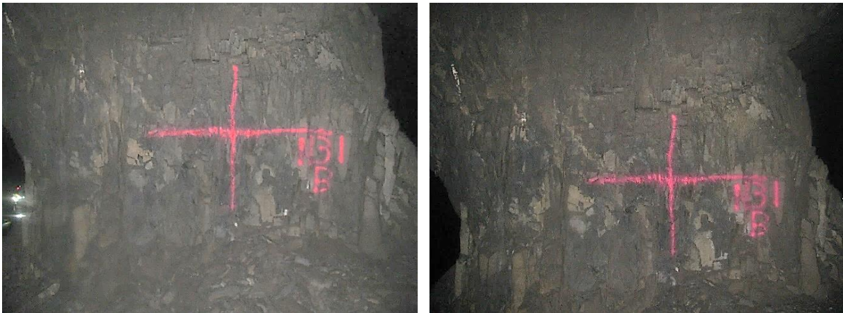
Figure 3-5. Measurement point painted on pillar N3_1 at Nchwaning III shaft. The photograph on the left was taken on 6 May 2021 and the photograph on the right on 18 August 2021. The lines were still pristine on the second date and no scaling occurred during this three-month period.
