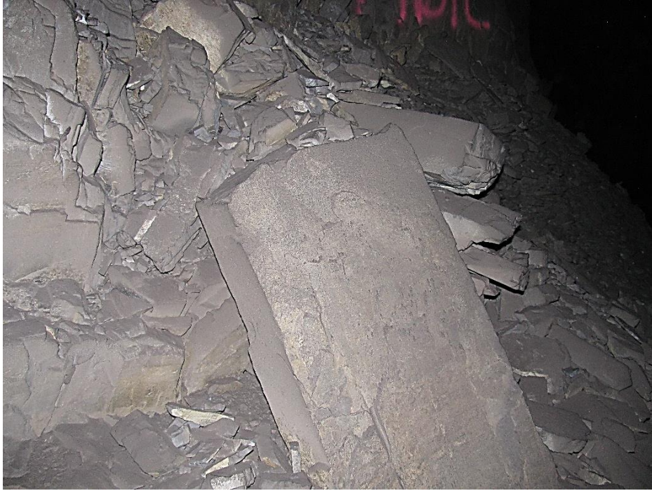
Figure 12-9. Side C of pillar N3_1 illustrating the size of some of the blocks that scaled from the pillar.
