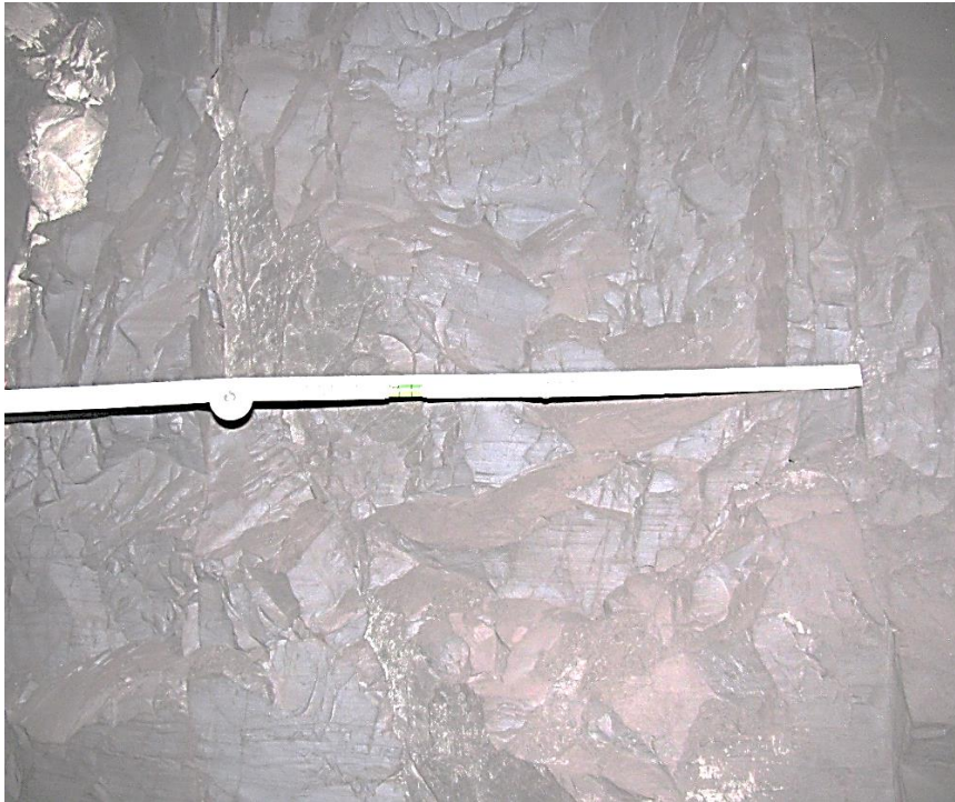
Figure 12-87. Side A of pillar N3_38 at Nchwaning III shaft, illustrating the vertical joint spacing of the pillar.
