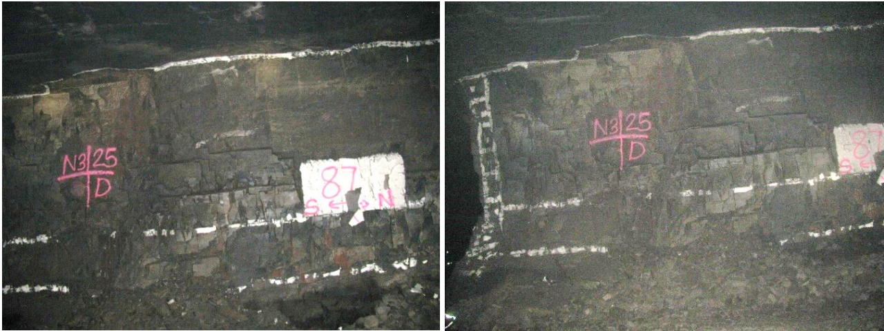
Figure 3-8. Pillar N3_25 at Nchwaning III Shaft. The photograph on the left was taken on 6 May 2021 and the photograph on the right on 18 August 2021. The broken white lines give an indication of a time-dependent scaling process, but this occurred prior to the monitoring done for this study.
