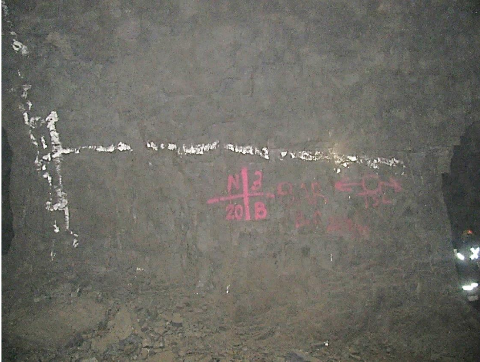
Figure 12-49. Side B of pillar N3_20 at Nchwaning III shaft as observed on the 18th of August 2021.
