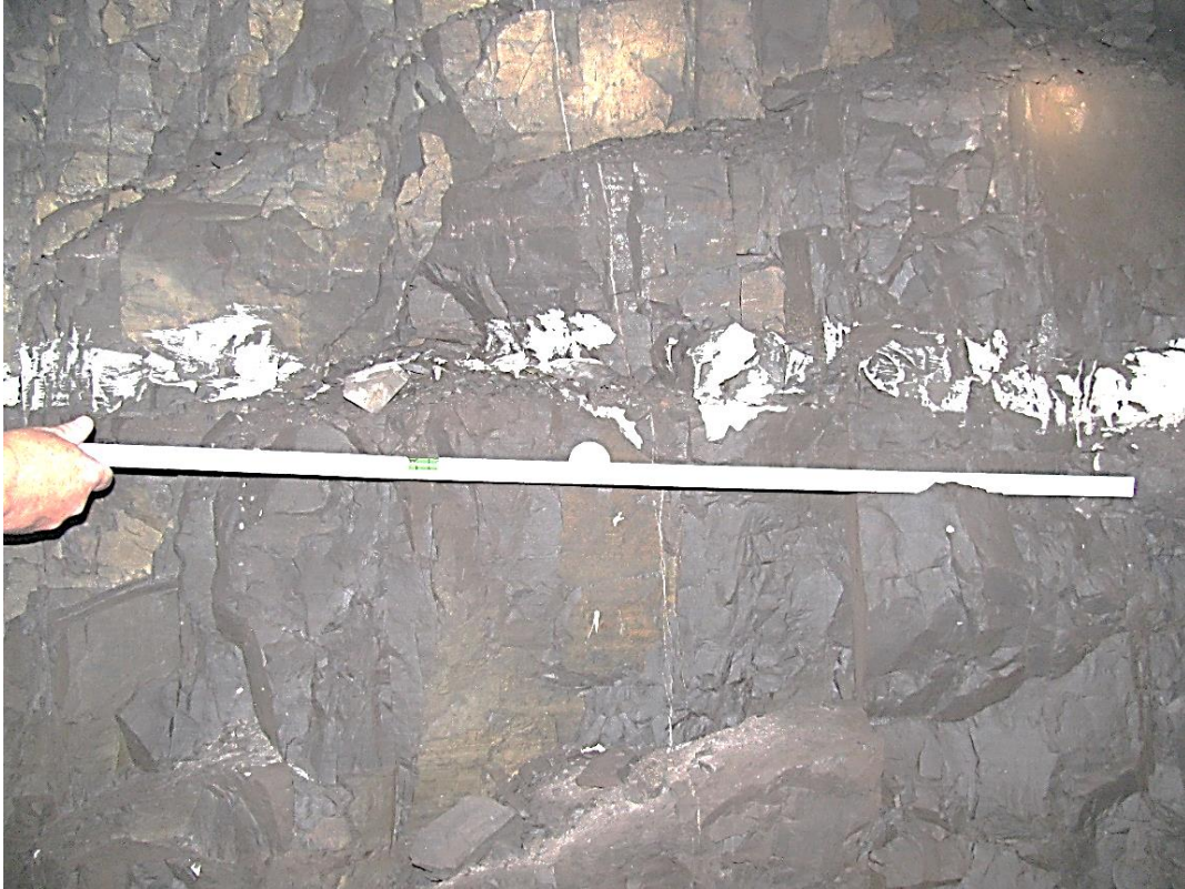
Figure 12-39. Side B of pillar N3_15 at Nchwaneing III shaft, illustrating the vertical joint spacing.
