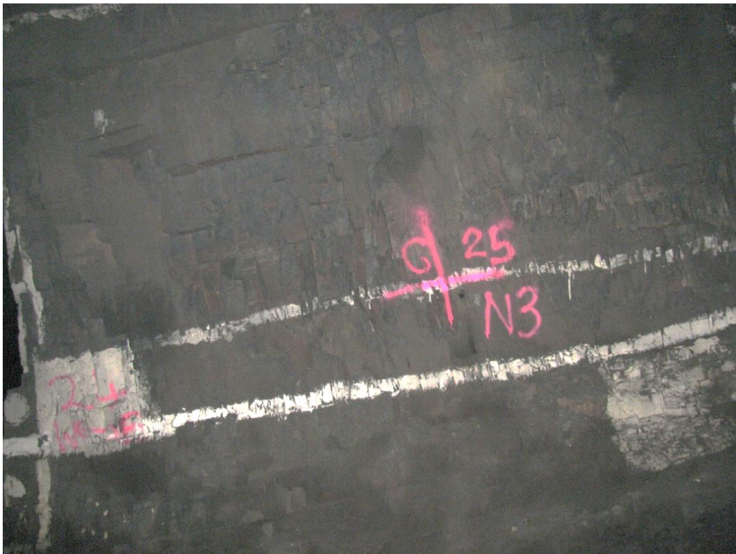
Figure 12-64. Side C of pillar N3_25 at Nchwaning III shaft as observed on the 6 th of May 2021.
