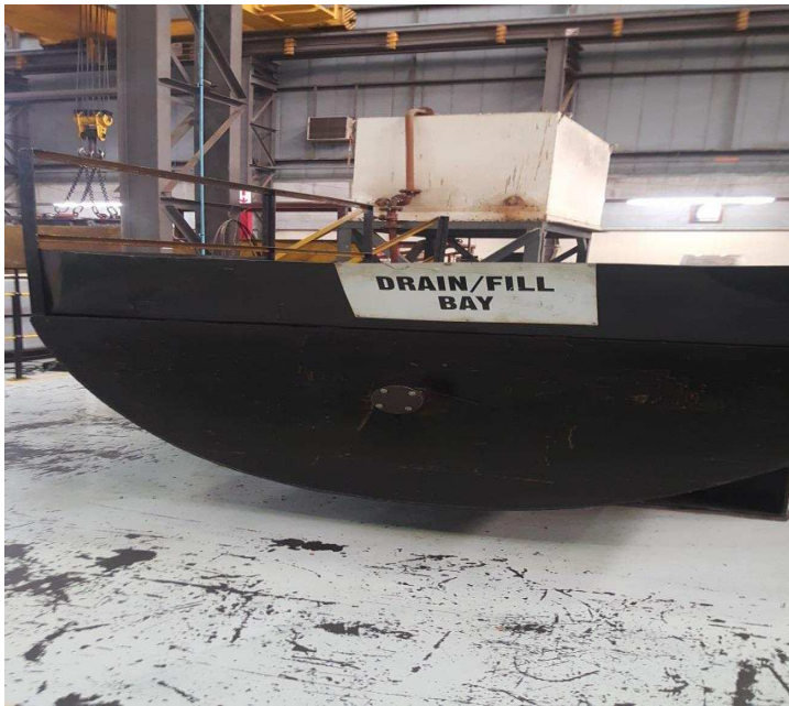
Figure 4.2: Drain Bay to contain the drained oil from the transformers for recycling – PPM Workshop - Witbank (Source: Author's own)
