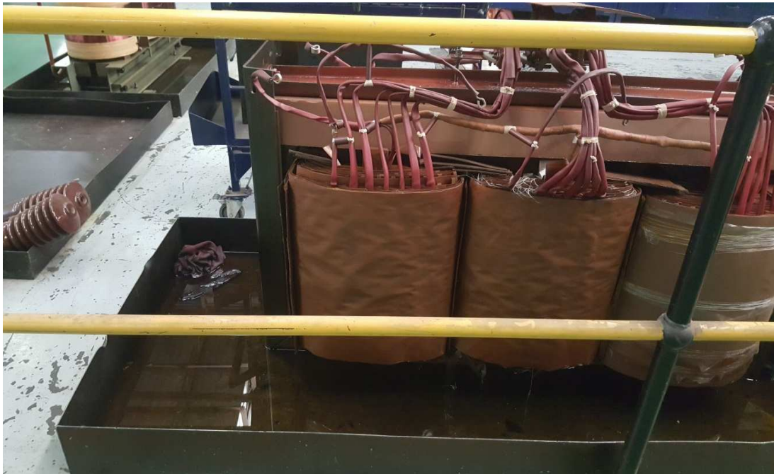
Figure 4.1: Power Plant Maintenance Workshop (PPM), Witbank – Maintenance area indicating transformers in an oil tray, to contain oil leaks from the transformer.
