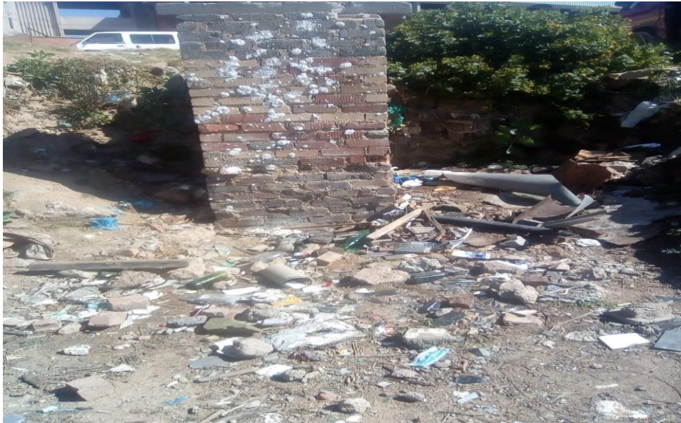
Photo P1(3): Environmental risk: Inadequate sanitation
