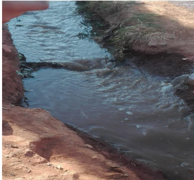
Photo P2(3): Environmental risk: Prolonged time to fix burst sewerage pipes
