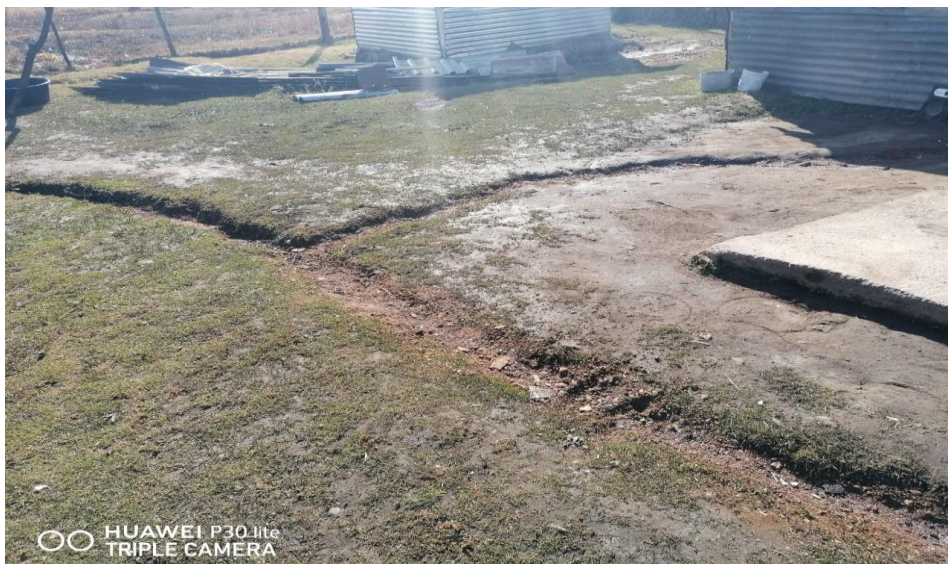
Photo P5(3): Poverty: Burst and unfixed water pipes
