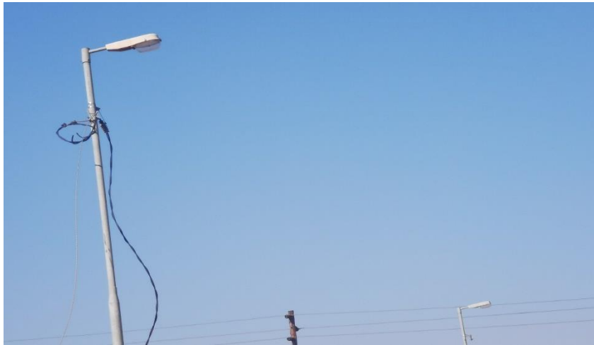
Photo P3(2): Poverty: Cable theft leading to non-functioning streetlights
