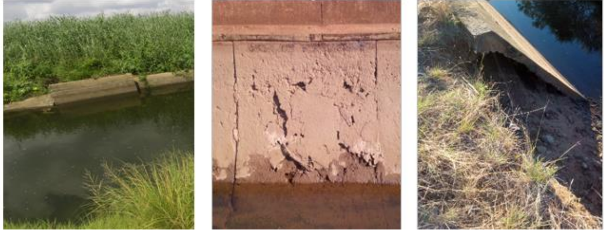
Figure 2-12: Canal lack of maintenance (DWS, 2016)
