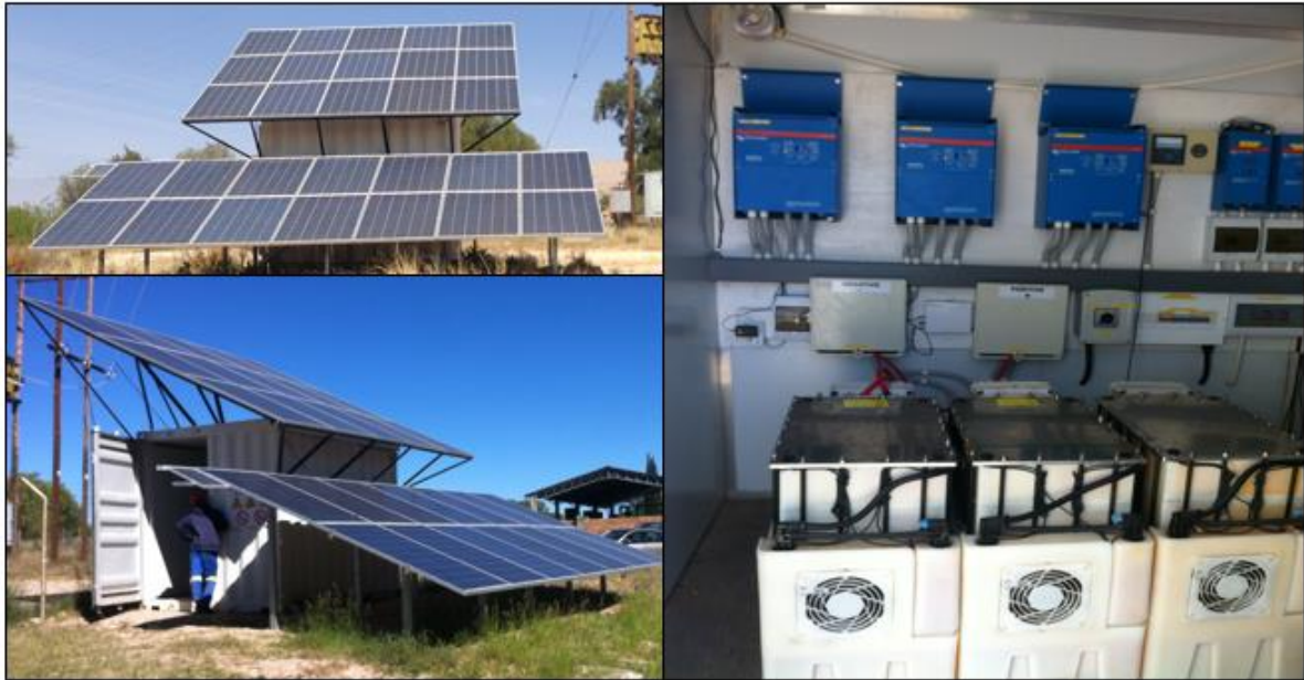
Figure 3-20: Existing solar plant
