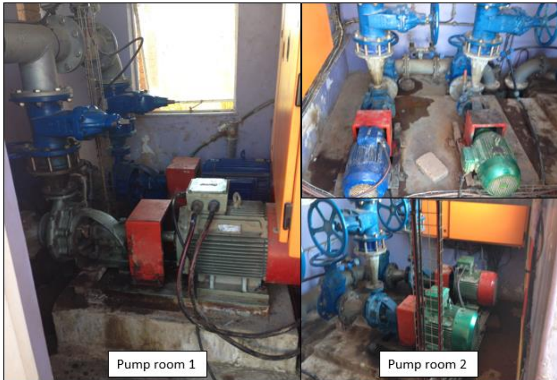
Figure 3-19: Pump station room 1 and 2
