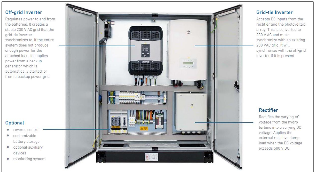
Figure 3-23: Electrical management system (Control panel) (SHP, n.d.)
