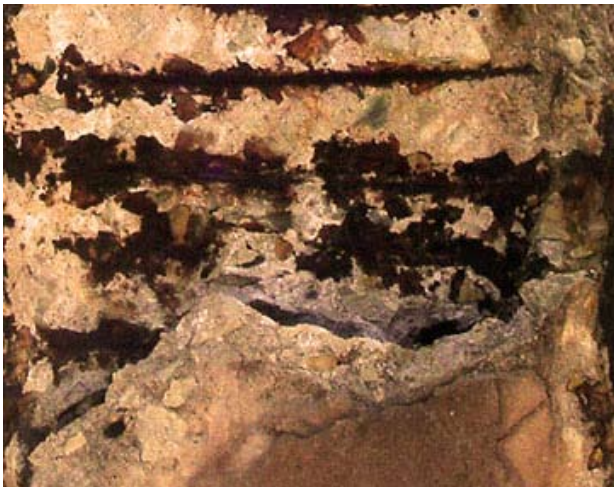
Figure 5.05 Corroded reinforced concrete storage tank structure [March 2009]
