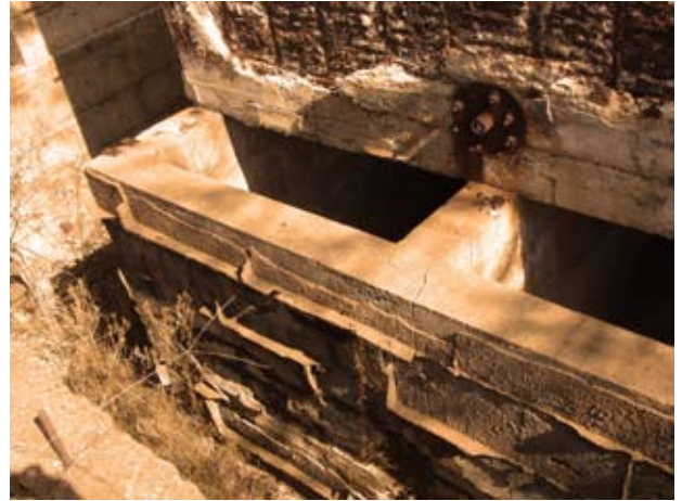
Figure 5.22 Reinforced concrete storage tanks [March 2009]
