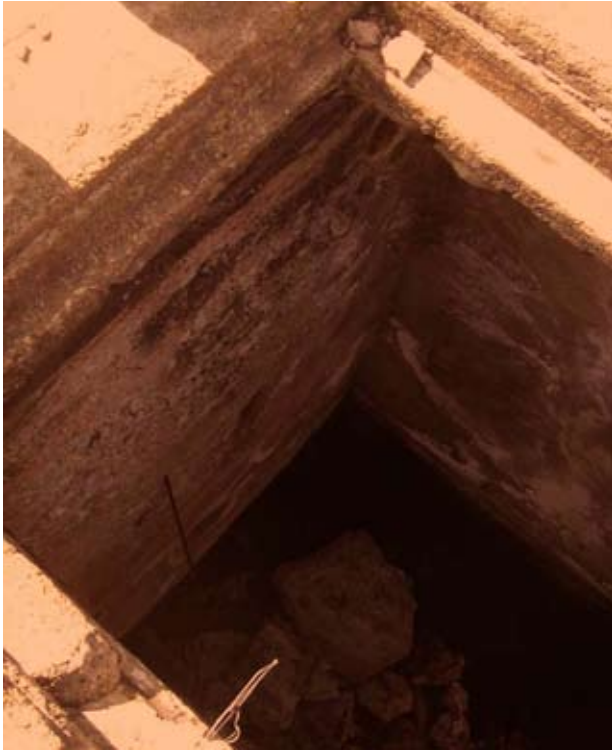
Figure 5.11 Dilapidated reinforced concrete storage tanks filled with rainwater
