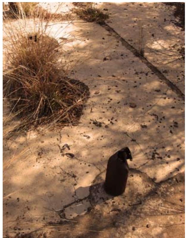
Figure 5.18 Concrete floor with corroded pipe elements protruding [August 2009]
