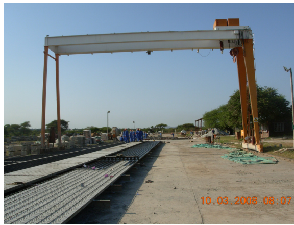
Figure 22 - Overhead Crane and Lintel Production Line
