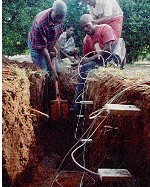
Figure 2.11. Installing HDS and TDR sensors in clementine hedgerow at Syferkuil.
