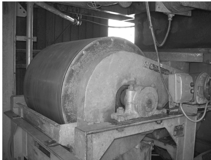
Figure A.7. The demagnetizing coil at the DMS plant.
