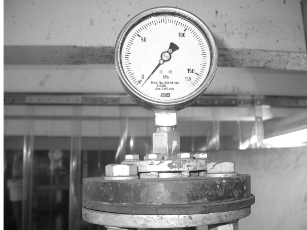
Figure A.2. The pressure gauge used to measure the feed pressure.
