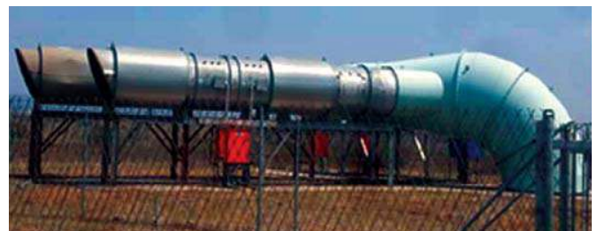
Figure 1: Photograph showing current 110 kW fan installation
