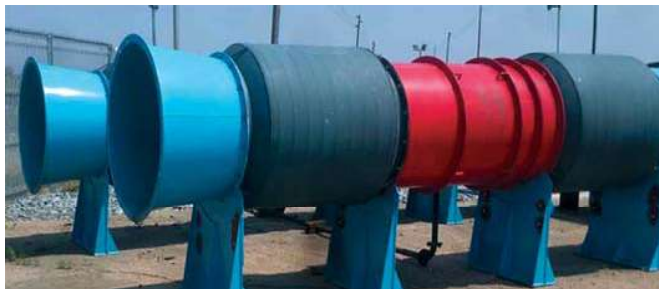
Figure 2: Photograph showing new fan installation
