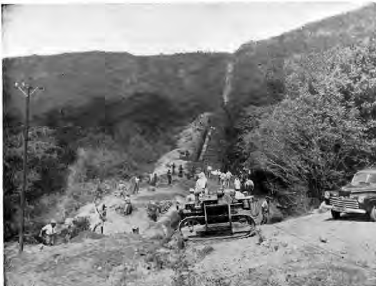
Digging for and laying the pipe over the extremely rough intervening country.
