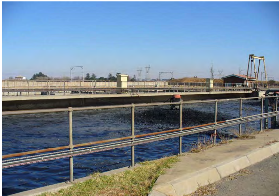
Figure 3.1. Aeration basin at the Leeuwkuil water purification plant. Biofilms were removed from the side of the aeration basin, 60 cm below the water level.
