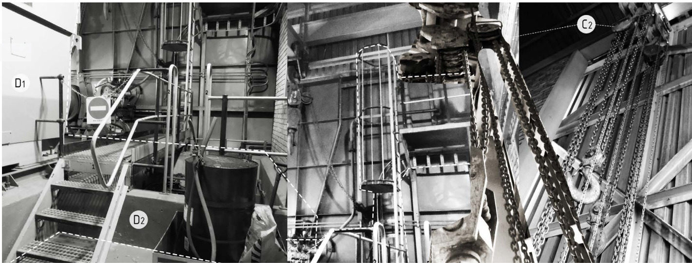
Figure 4.28 Inside the motor rooms (Author, 2014)
