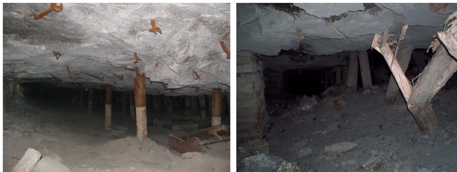
Fig. 2. Photographs of a typical tabular platinum stope (left) and the hanging wall unravelling along the joints prior to a large panel collapse (right). There are many interacting blocks in the hanging wall. Note the evidence of significant closure and the broken elongates.
