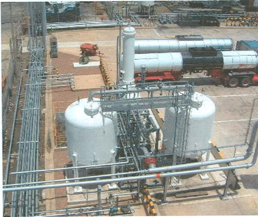
Figure 3.7 Vapour recovery unit at Engen-Wentworth, Durban.
