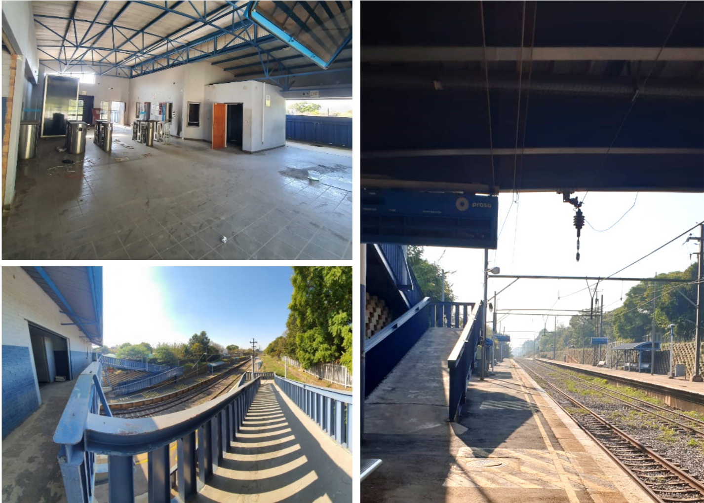
Figure 77 | Existing Train Station. Left: Ramp and underside of existing floor plate. Top Right: Existing Floor plate. Bottom Right: Existing Ramps and part of Floor plate.
