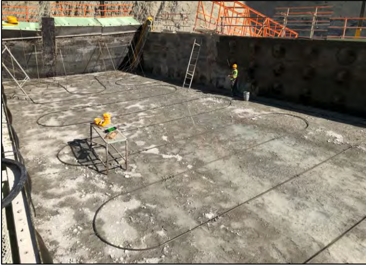
Figure 3-21: Pipes placed in coil formation on top of old lift for post cooling of concrete in subsequent lift
