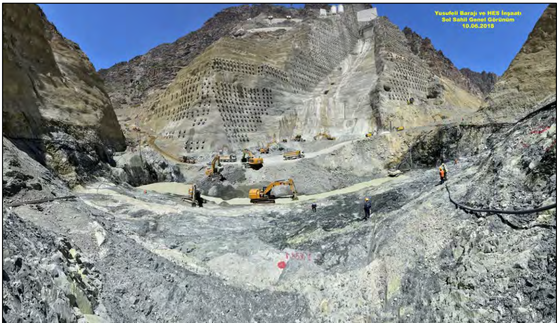
Figure 3-13: Wide angle view of the final stages of excavation at the deepest foundation point in the river basin
