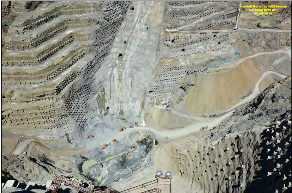
Figure 3-12: Final stages of excavation at the deepest foundation point in the river basin
