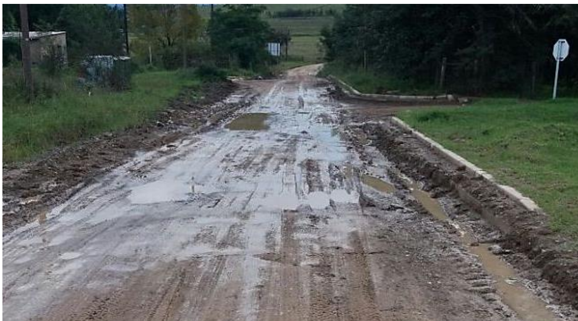
Figure 2-4: Deterioration of an unpaved road in wet conditions (Rnews.co.za, 2018)
