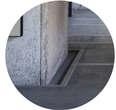
GAP HIGHLIGHTED WITH RECESS BETWEEN OLD WALL AND NEW FLOOR
