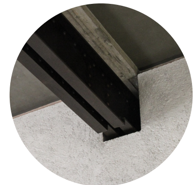
NEW STRUCTURAL STEEL MEMBER IS STEPPED TO CREATE A RECESS THAT RESPECTS THE OLD WALL
