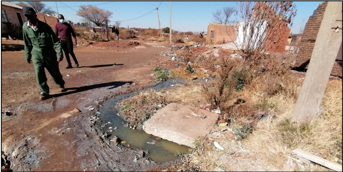
Figure 43: Broken, blocked and back ponding sewer line at Adatite Street, Khutsong Proper.
