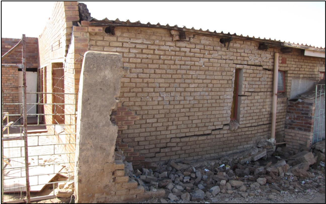
Figure 39: A subsidence forming against the house casing a severe wall distress, Khutsong Extension 3.
