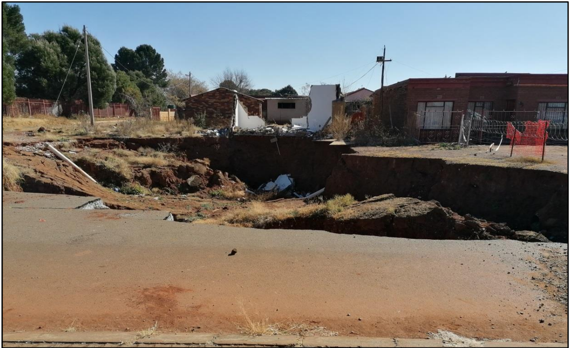
Figure 22: A very large sinkhole (>15m diameter) at Nxumalo Road, Khutsong Proper.
