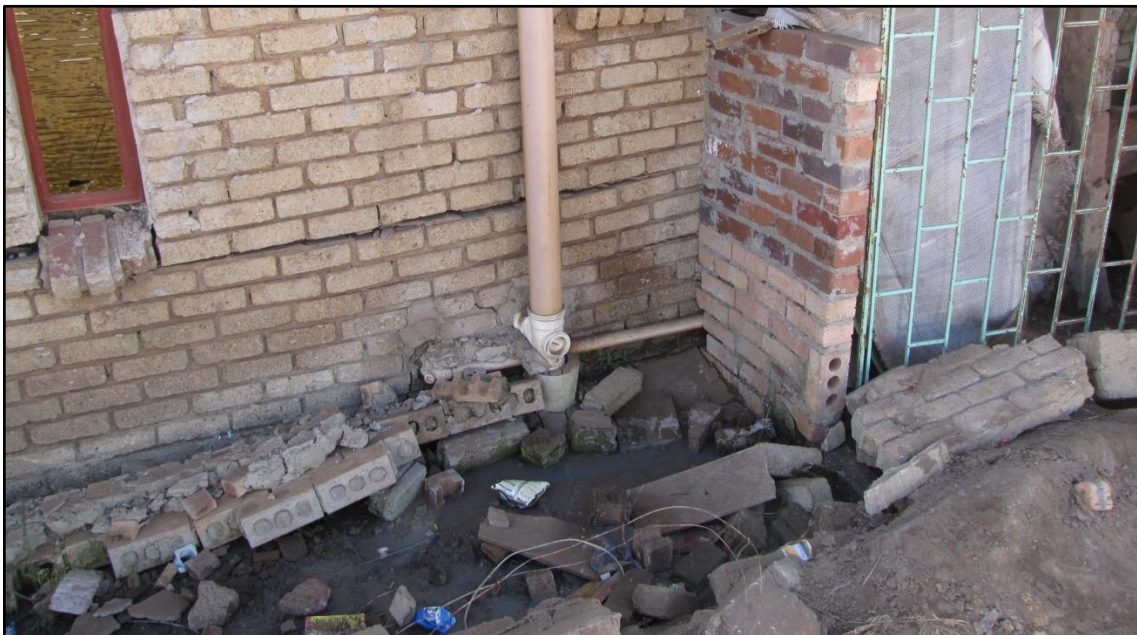
Figure 40: Sewage damming against the wall, Khutsong Extension 3.
