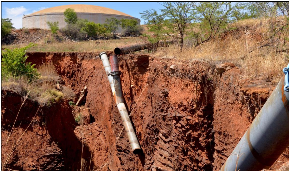
Figure 42: Damage to a bulk water supply pipeline, Carletonville area.
