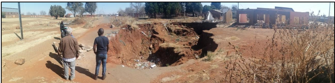
Figure 37: A very large sinkhole causing damage to main Nxumalo Road, Khutsong Proper.
