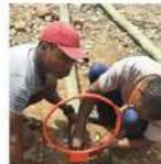
Through practical application with some supervision handy work is taught through an experiential approach to construction.
