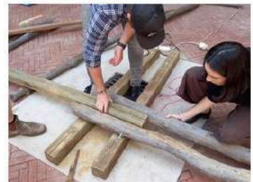
A prototype built by the Morelets Park Integration Project to develop a method of constructing with uneven elements (MPIP, 2021).
