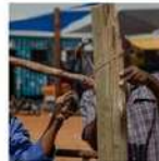
Through practical application and previous experience a house is built from materials found on site.
