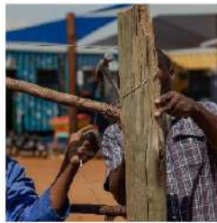
Through practical application and previous experience a fence is built from materials found on site.
