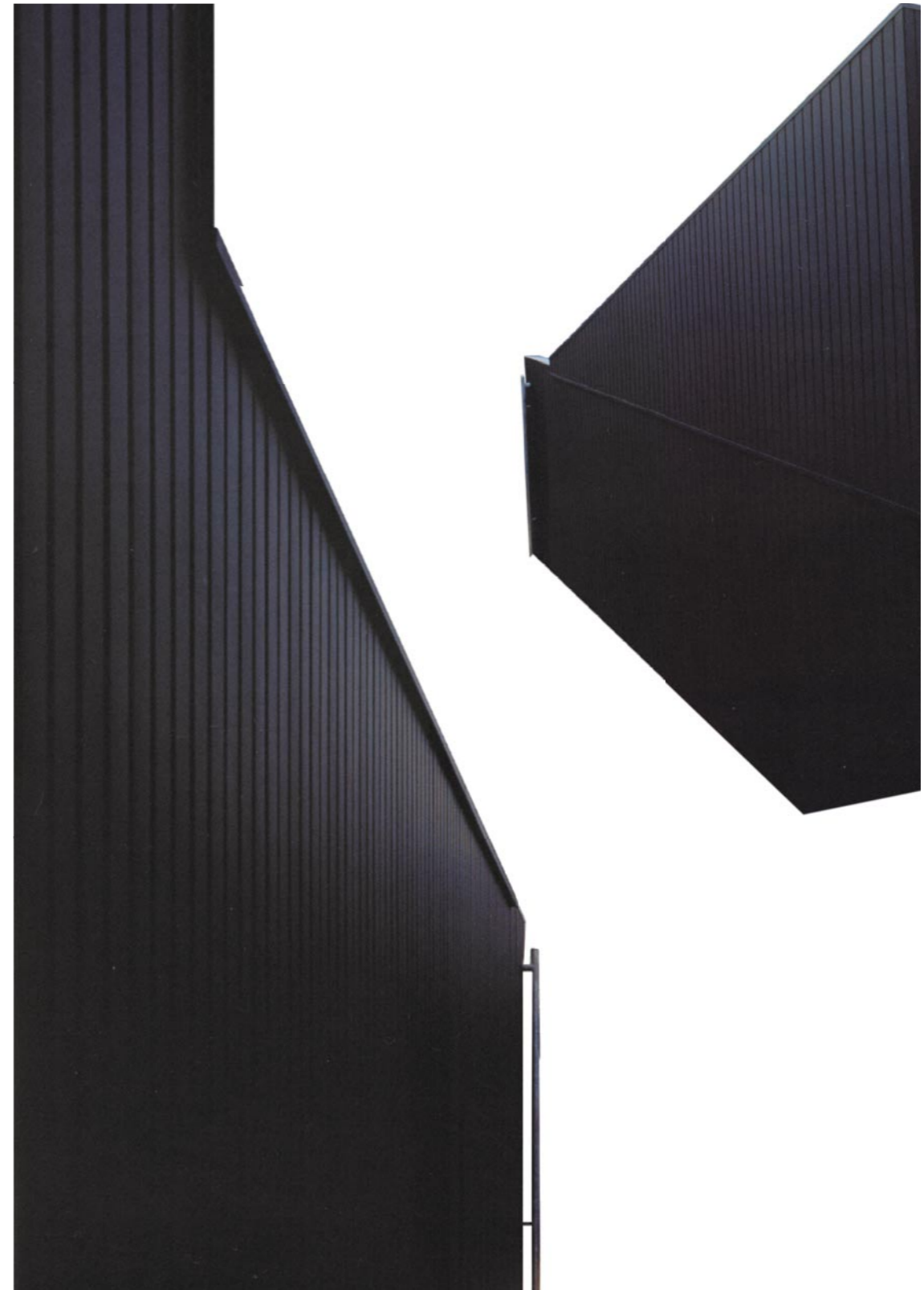
Fig 115 Powder coated black intumescent paint on steel sheeting. Waro Kishi & K. Associates, Hu Tong Private residence, 2002, western Japan. (Hadid, Z. Forster, K. Sudjic, D. et al. 2005: 398 - 399)
