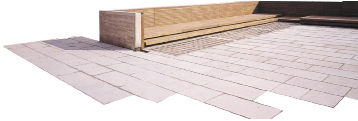
Fig. 116 Pre-cast concrete block floor. Atelier Barani, Youth Studio at the concrete art centre, 1997-1998, Mouans-Sartoux, France. (Hadid, Z. Forster, K. Sudjic, D. et al. 2005: 46 – 47)
