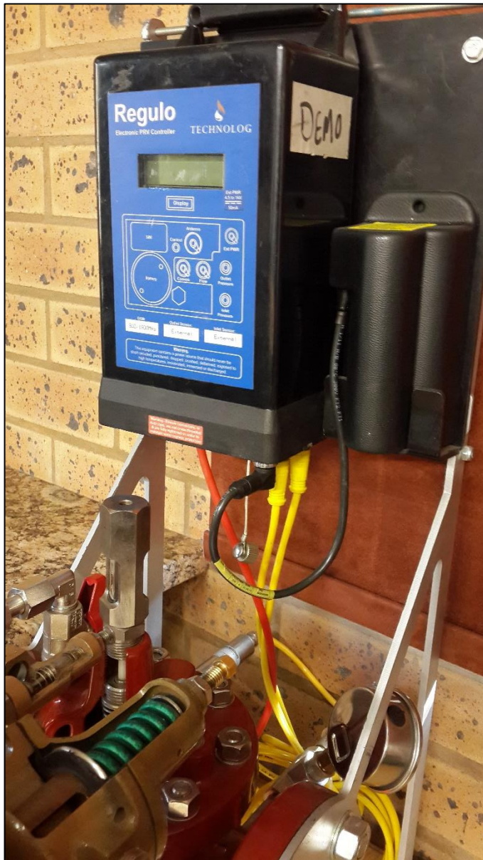
Figure 11. Pressure Reducing Valve (Photo was taken at WRP Consulting in Pretoria, 5 th July 2019).
