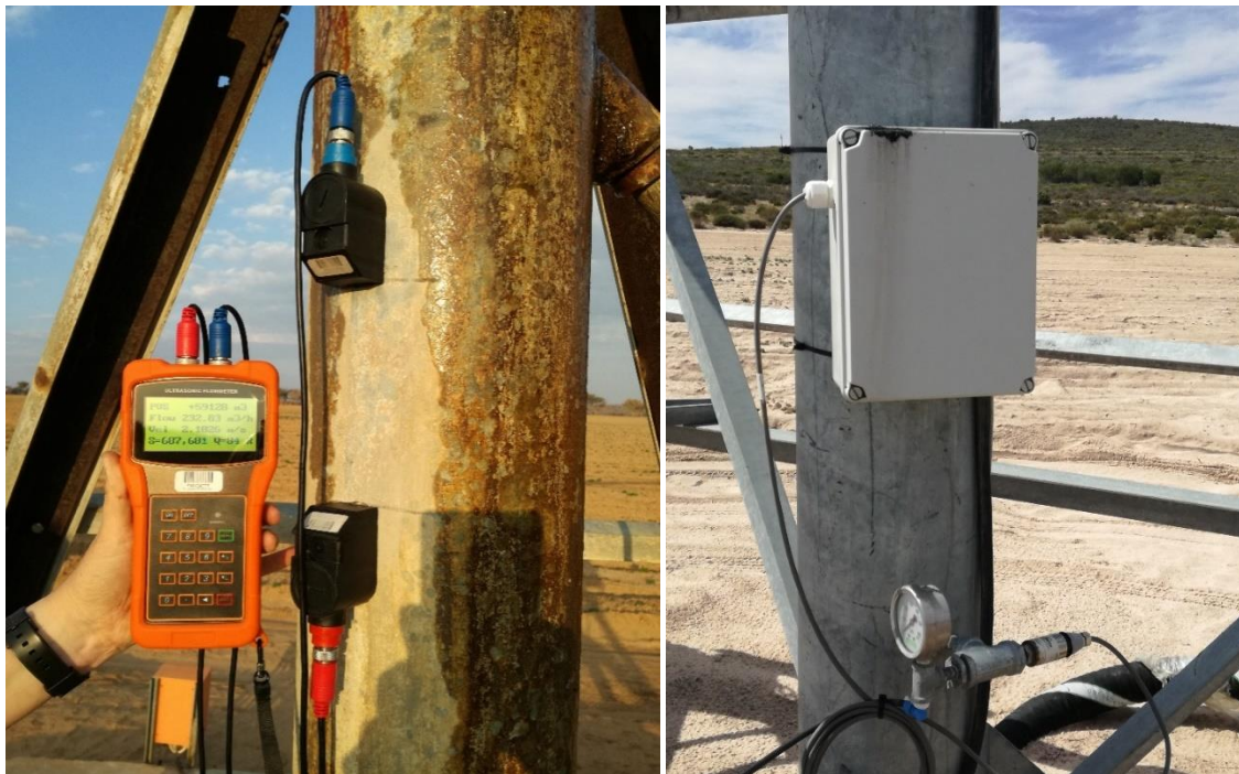
Figure 3-3: Ultrasonic flow meter (left) and pressure transducer with CR300 data logger (right) installed on a centre-pivot system.
