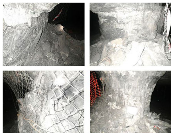
Figure 7—A Class 5 failed pillar in the pillar project area
