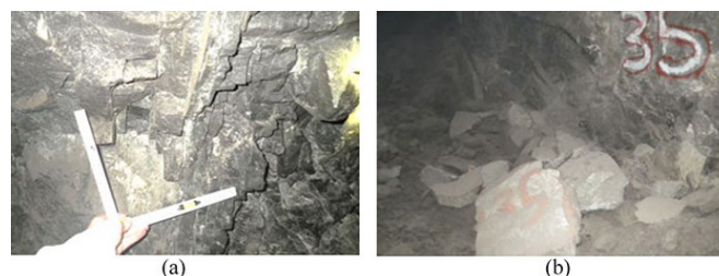
Figure 10—(a) An example of closely spaced joints sets found for the geologically disturbed pillars. (b) Scaling along the multiple joint sets observed in the areas near potholes
