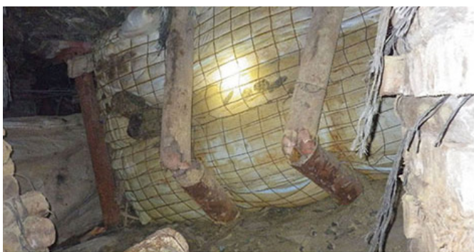
Figure 6—A backfill paddock in a deep tabular gold mine. The stope closure compressed the backfill and the lateral dilation broke the elongates used to construct the paddock
