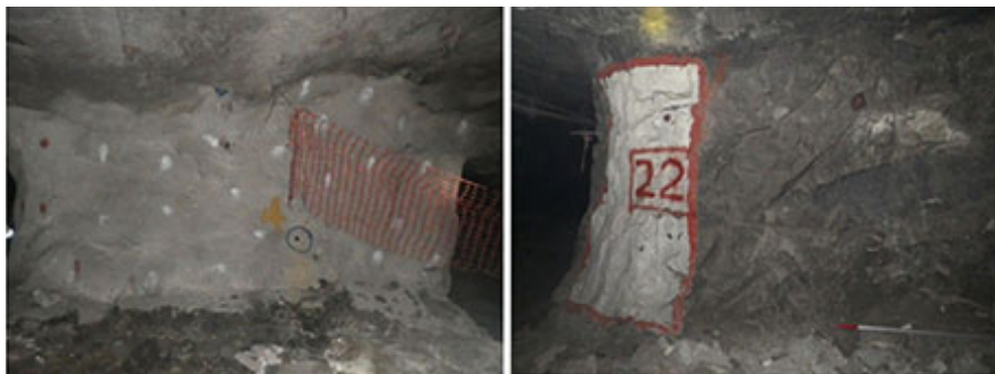
Figure 15—Condition of a rehabilitated pillar in the area of interest (left). Only a few pillars were covered with shotcrete. The photograph on the right illustrates the general condition of the pillars in this area
